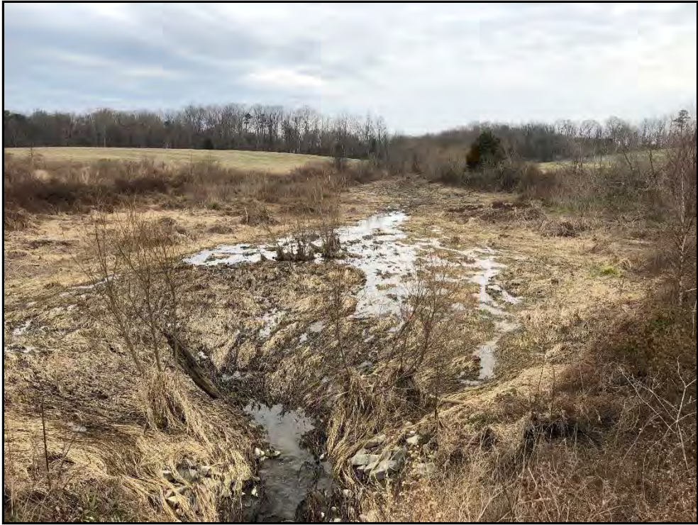
Project Reach UT2-2– Permanent Photo Station 11 Station 11+00 – Looking Upstream at Pond Bottom January 2019
