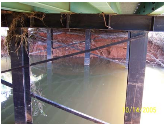
Debris hanging under bride.
