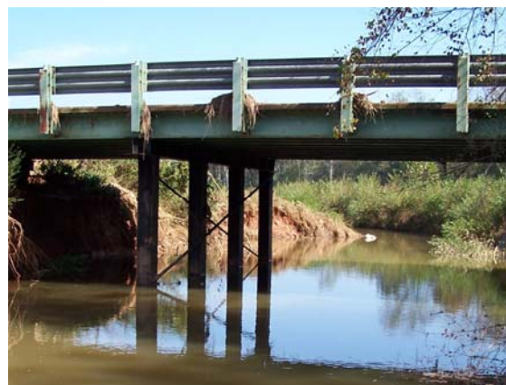
Debris hung on railings of the bridge.
