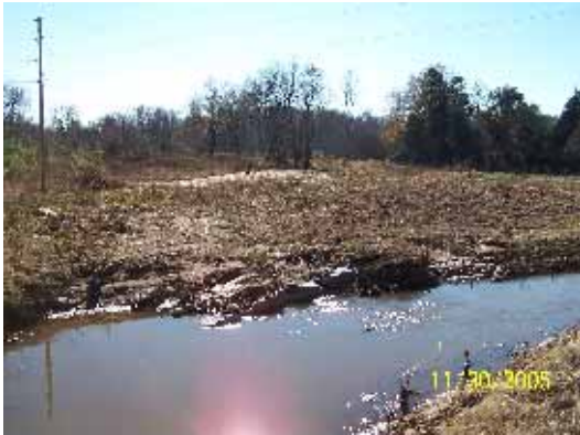
Silt deposition and minor scour at rock vane downstream of bridge.
