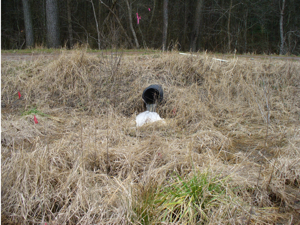
Inflow from upstream watershed in February. Vegetation too thick to show flow.
