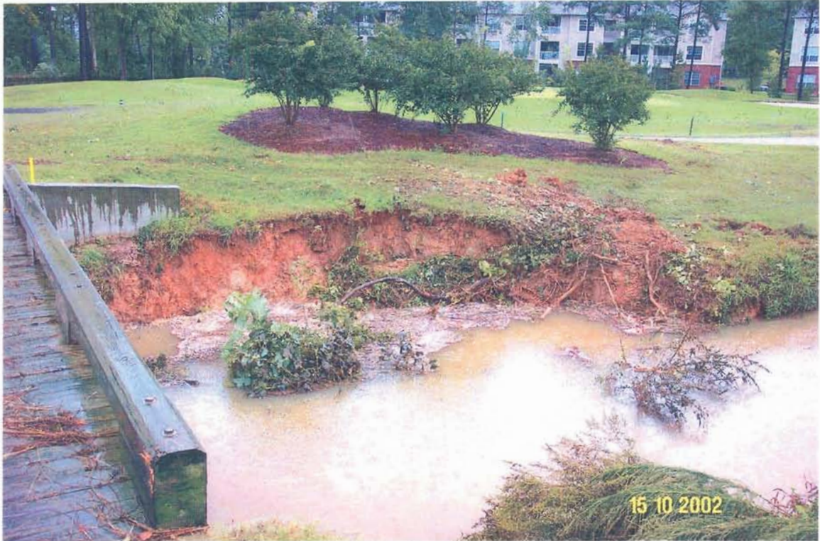
Ongoing bank erosion above bridge #3 after high flow (note collapsed vegetation)
