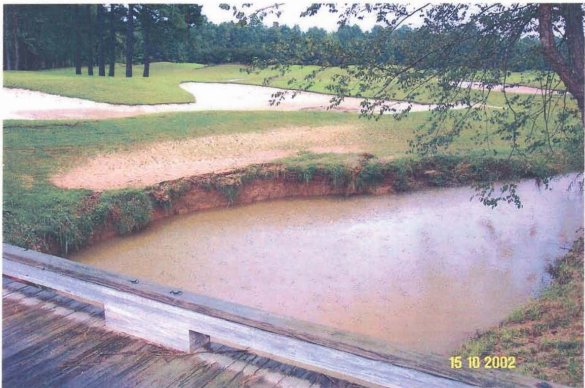
Bare, vertical bank with high erosion potential at high flow
