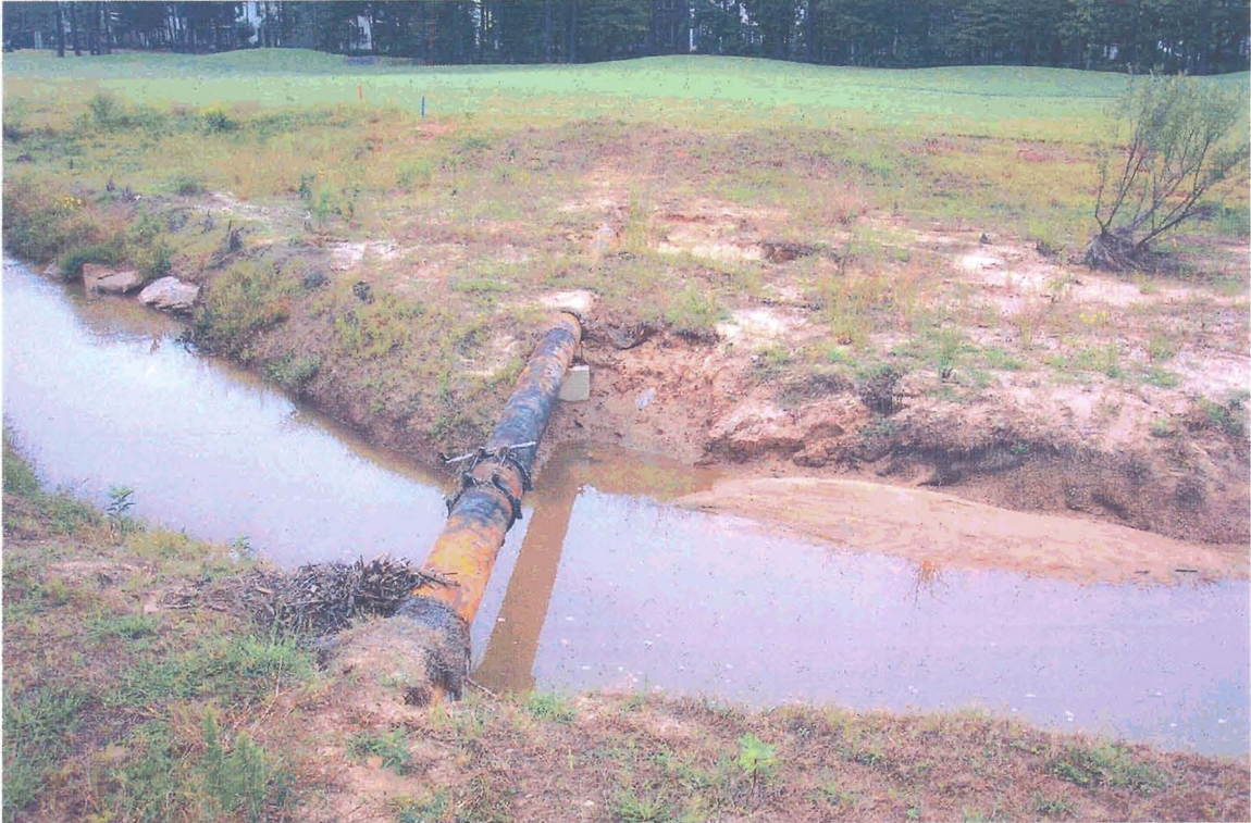
Bank Scour Located Immediately Below Sewer Pipe
