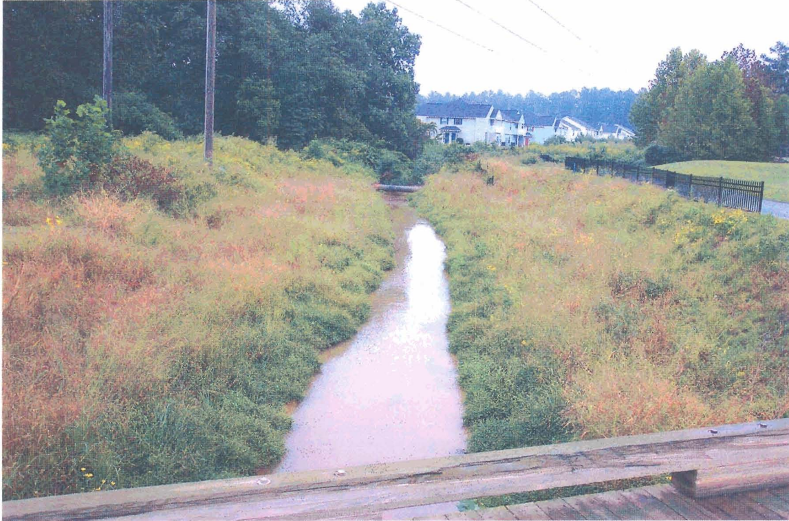
Lower 300 feet of Restoration Oriented Upstream; Sewer Pipe is the Project Terminus
