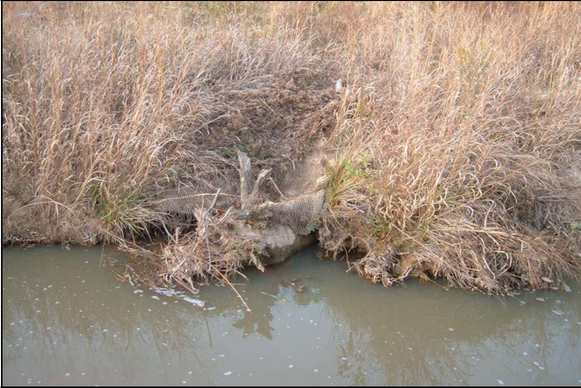
SP3 – Scour around rootwad. Vegetation and coir matting partially obscure the erosion behind the rootwad. Photo taken near station 29+10. 11/5/06 - MY 02
