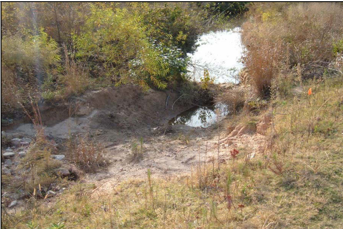
SP2 – Severe bank erosion and floodplain scour. Photo taken near station 14+75, looking down on an eroded bank and a scour hole in the floodplain. 11/5/06 - MY 02
