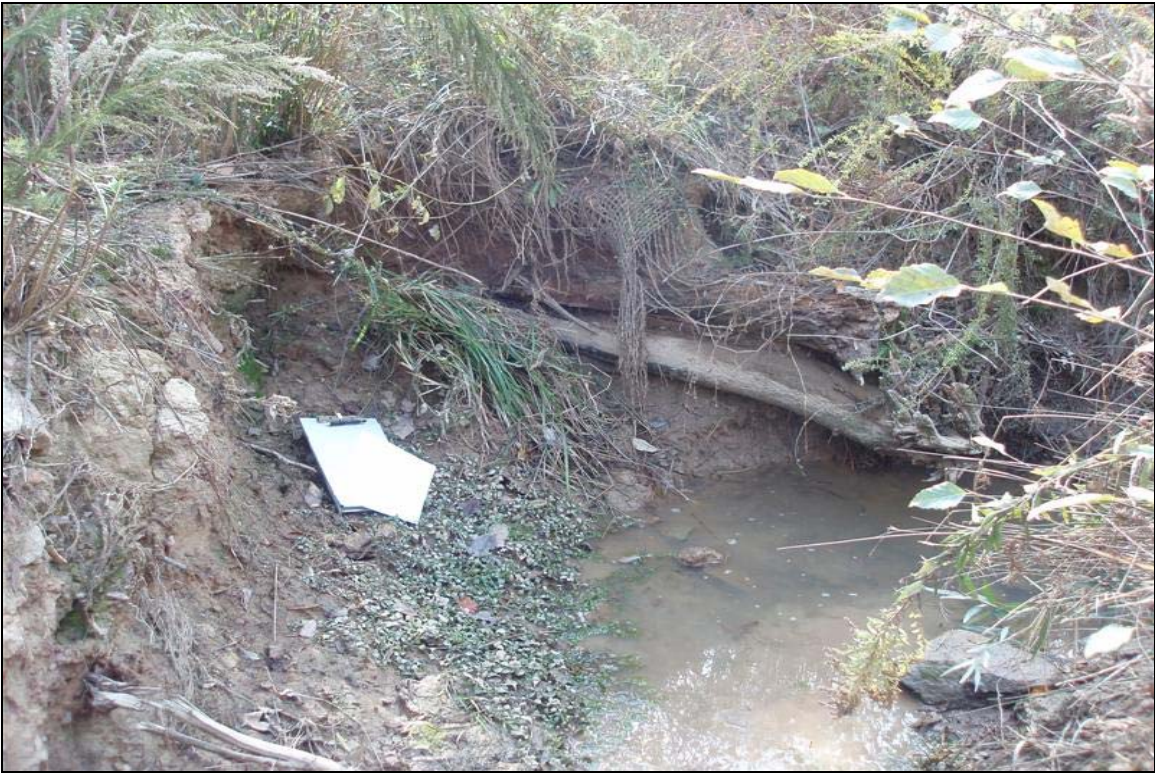
SP7 - Back scour around rootwad and bank erosion. Rootwad partially obscured by coir matting. Photo taken near Station 02+10. 11/13/07 - MY 03
