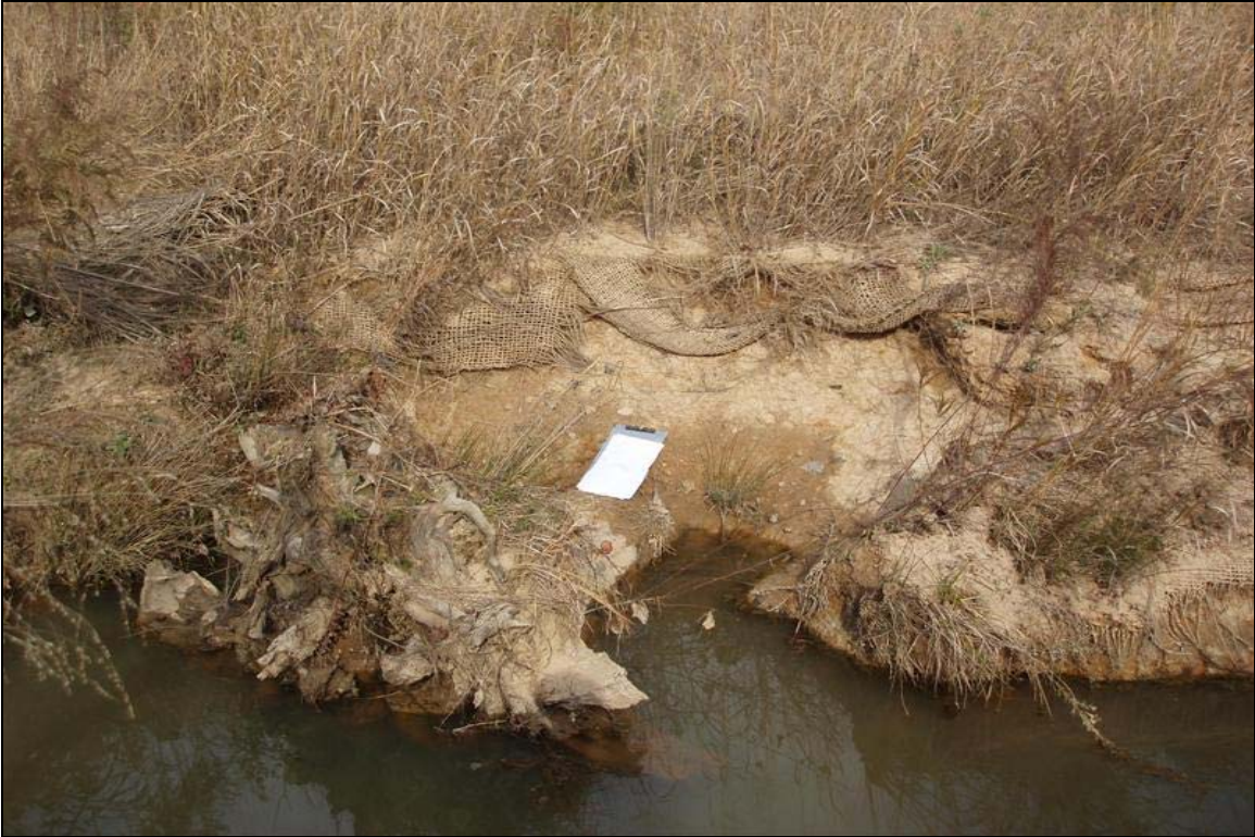
SP3 - Scour around rootwad. Vegetation and coir matting partially obscure the erosion behind the rootwad. Photo taken near Station 37+50. 11/13/07 - MY 03
