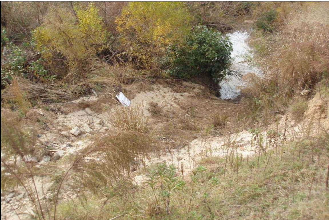
SP2 - Severe bank erosion and floodplain scour. Photo taken near Station 14+75, looking down on an eroded bank and a scour hole in the floodplain. 11/13/07 - MY 03
