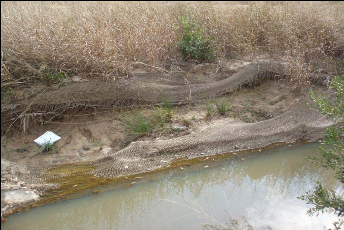
SP1 - Bank erosion. Photo taken near Station 18+60. 11/13/07 - MY 03
