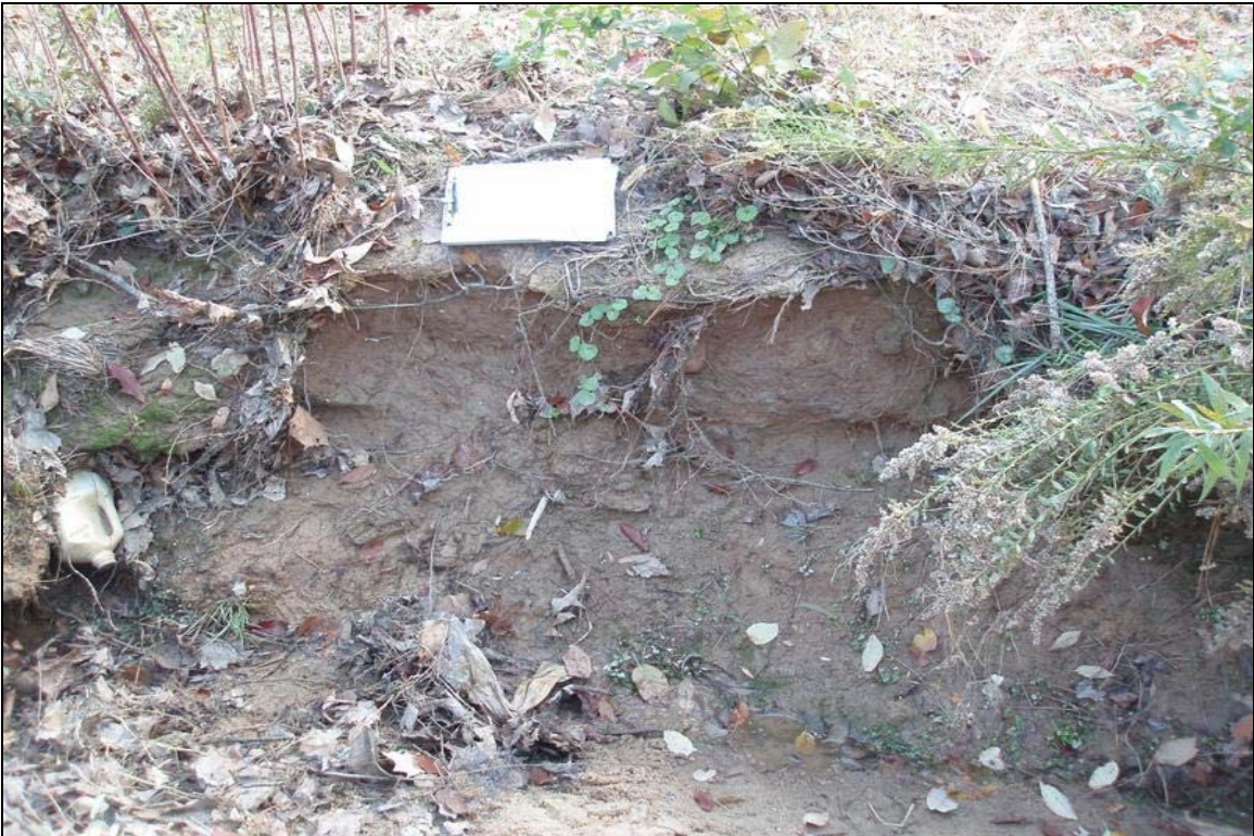
SP6 - Bank erosion. Photo taken near Station 00+75. 11/13/07 - MY 03
