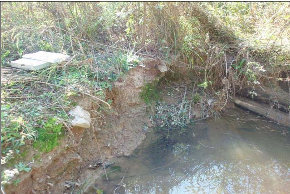
SP6 - Bank erosion. Photo taken near Station 2+00. 10/27/08 - MY 04.
