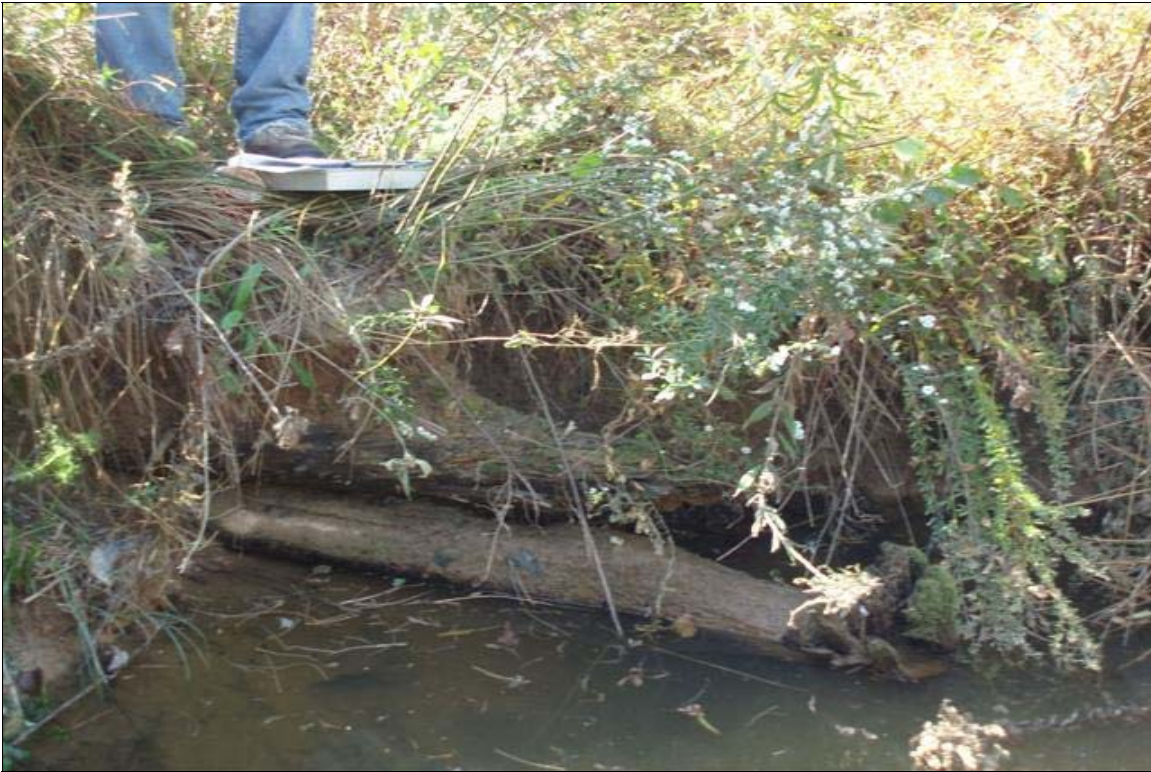
SP7 - Back scour around rootwad and bank erosion. Rootwad partially obscured by coir matting and vegetation. Photo taken near Station 02+10. 10/27/08 - MY 04.
