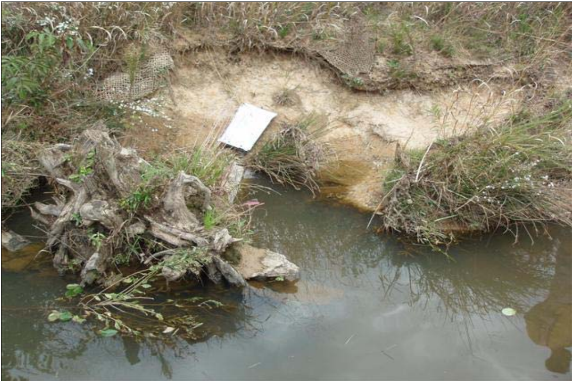
SP3 - Scour around rootwad. Photo taken near Station 37+50. 10/27/08 - MY 04.
