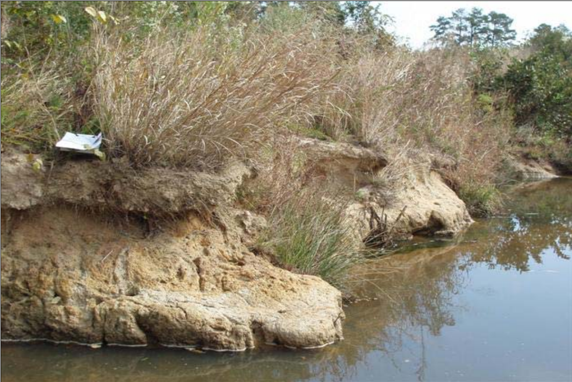
SP1 - Bank erosion. Photo taken near Station 18+60. 10/27/08 - MY 04.
