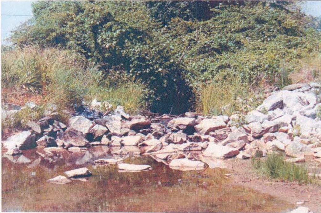
Picture 17. View of stream from inside box culverts looking upstream after road construction.
