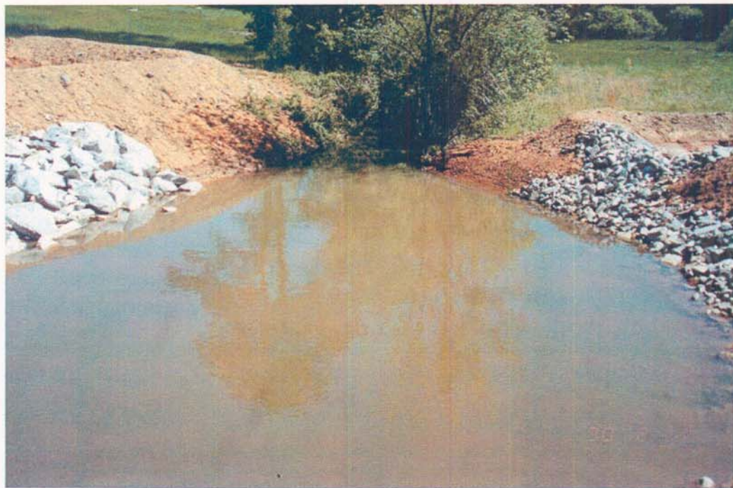
Picture 16. View of stream from inside box culverts looking upstream during road construction.
