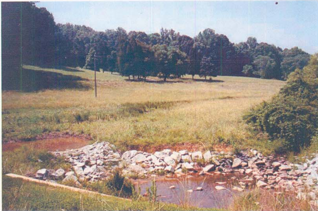
Picture 13. On Hobbs Road, box culverts looking upstream after road construction was complete.
