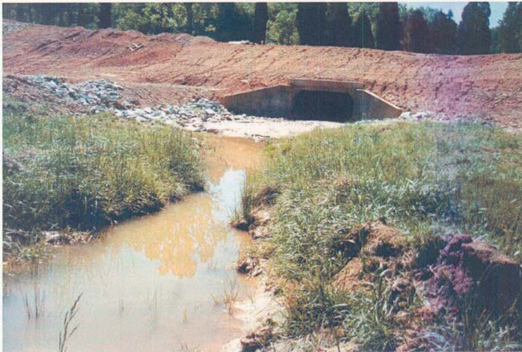
Picture 14. Stream disturbance during road construction looking downstream.
