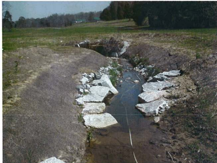
M5-DS: View from Meander 5 looking downstream towards Meander 6. Note the cross rock and the boulder adjacent to it on the right have settled since construction and are below the water surface.
