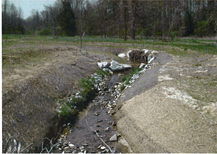
M6-US: View from Meander 6 looking upstream towards Meander 5. Note rip-rap was installed at the end of construction due to bed downcutting.
