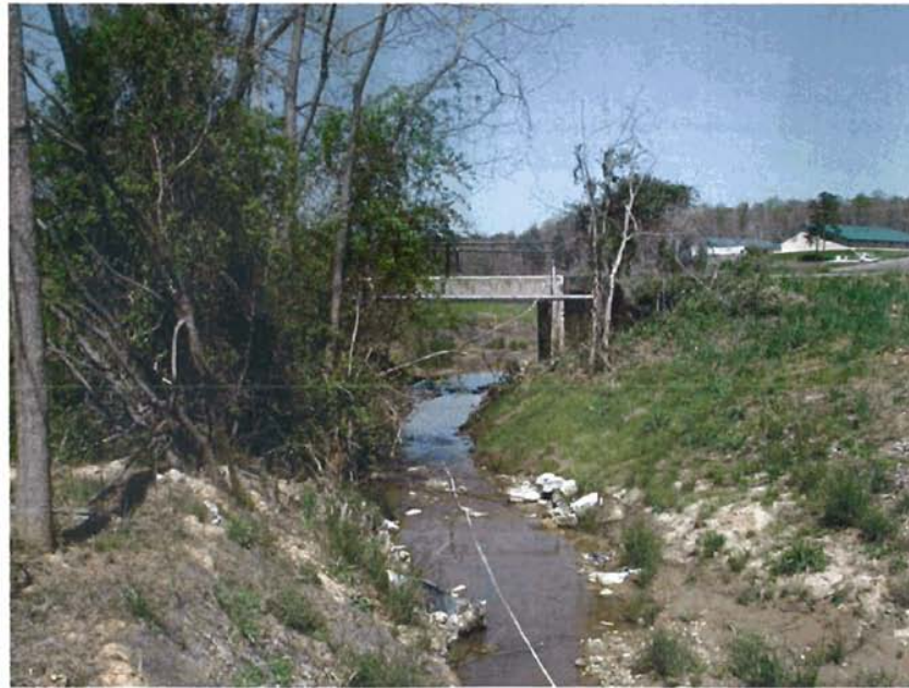
M11-DS: View from Meander 11 looking downstream. Jefferson Club Road crosses the stream via this 14' x 7.5 box culvert.
