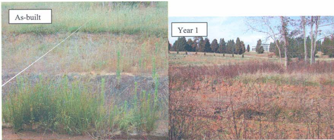
Transect 7 (BT7-L)– Left bank below bridge. Shows significant elevation change between build-out bench and buffer elevation.
