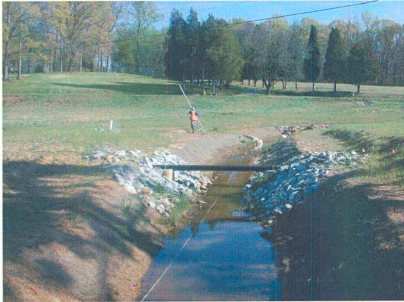
M16-US: View from Meander 16 looking upstream. The aerial sewer line was re-routed to make it perpendicular to the stream.
