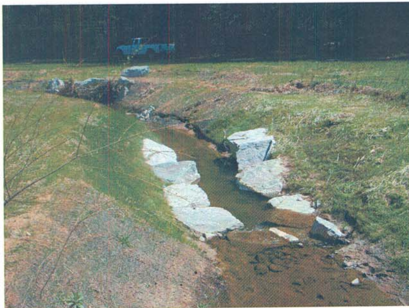
M3-DS: View from Meander 3 looking downstream towards a cross vane that was installed after the main construction period due to concerns with the grade downstream.
