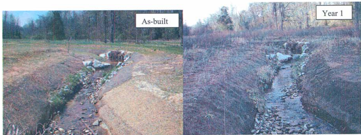
M6-US: View from Meander 6 looking upstream towards Meander 5. Note rip-rap was installed at the end of construction due to bed downcutting.
