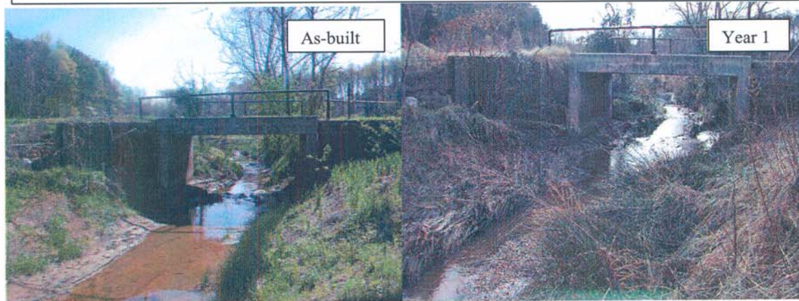
M12-US: View from Meander 12 looking upstream through the culvert. Note how the channel has narrowed and vegetated in the Year 1 photograph.
