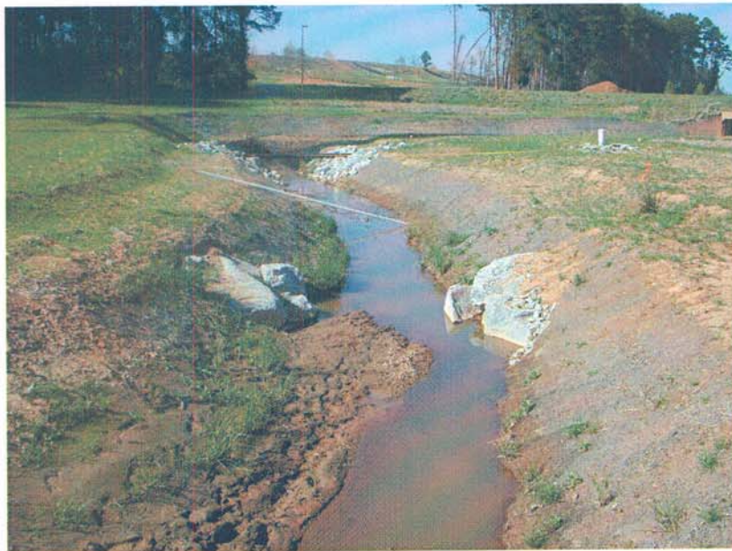
M15-DS: View from Meander 15 looking downstream. Note this cross-vane was moved upstream into the meander to avoid a gas line during construction. In effect, the upper portion of the cross vane has been covered up by the point bar since the cross vane slowed the water on the inside meander.
