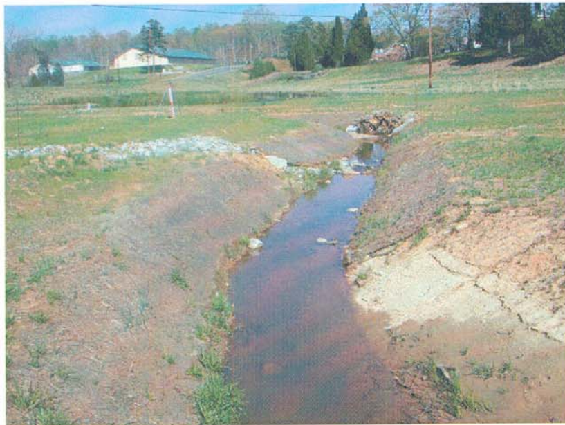
M14-DS: View from Meander 14 looking downstream. Note stone step-pool outfall to connect roadway drainage to stream.
