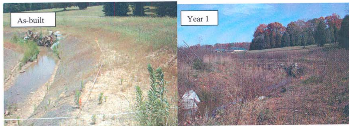
Transect 5 (BT5-D)– View of right build-out bench looking downstream. Note development of sedges and rushes on point bar above structure.
