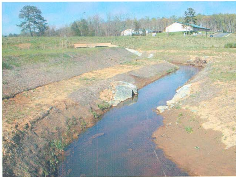
M16-DS: View from Meander 16 looking downstream. Cross-vane is drowned out due to backwater from the off-site lake downstream.
