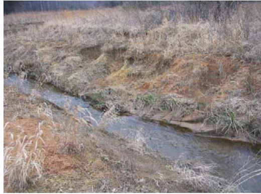
Issue Photo 8 – Station 8+50 Bank slump due to over-bank wash
