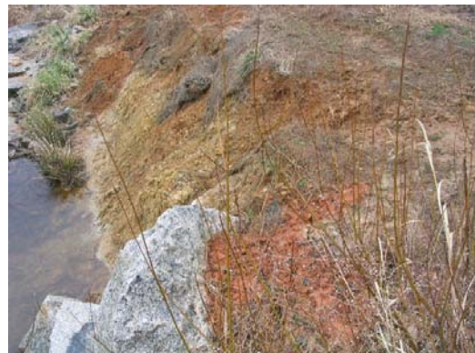
Issue Photo 4 – Station 5+00 Erosion on bank below cross vane and washed away matting
