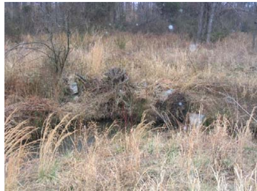
Issue Photo 2 - Station 3+60. Bank erosion behind rootwads.
