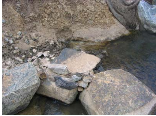
Issue Photo 6 – Station 6+00 Cutting under cross vane
