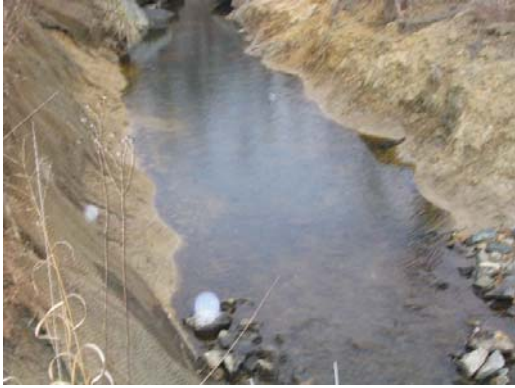
Issue Photo 5 – Station 6+50 Unprotected bank
