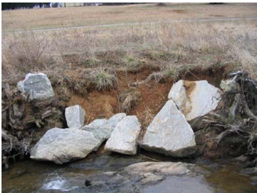
Issue Photo 9 – Station 13+70 Bank slump between root wads resulting from overland flow
