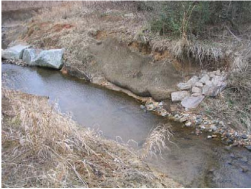
Issue Photo 7 – Station 7+40 Bank slump due to over-bank wash
