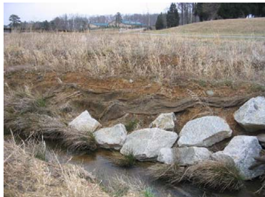
Issue Photo 10 – Station 14+10 Bank washout
