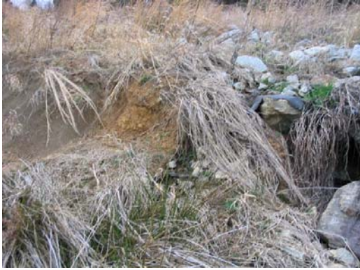
Issue Photo11 – Station 13+50 Erosion near drainage channel
