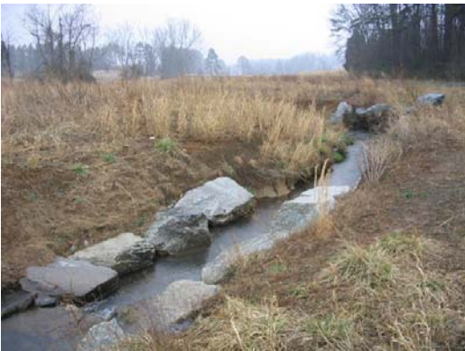
Issue Photo 1 - Station 3+00. Bank scour below cross vane
