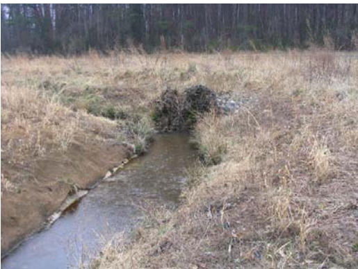
Issue Photo 3 – Station 5+30 Unsecured matting and unvegetated bank.
