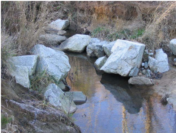
Issue Photo 4 - Station 2+10. Cross vane with footers undermined and boulders slumping
