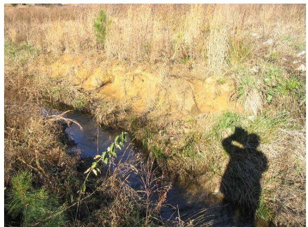
Issue Photo 12 - Station 15+50. Left bank un-vegetated with signs of scour from stormflow and overland flow
