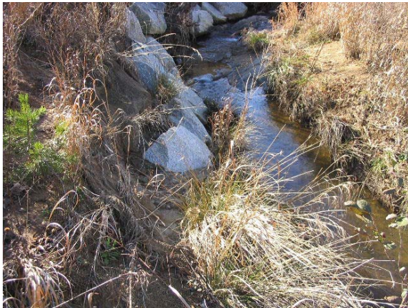
Issue Photo 9 - Station 6+80 Right bank scour and inadequate vegetation
