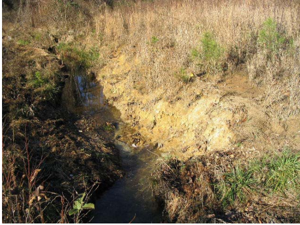
Issue Photo 1 - Station 0+80 Left bank un-vegetated
