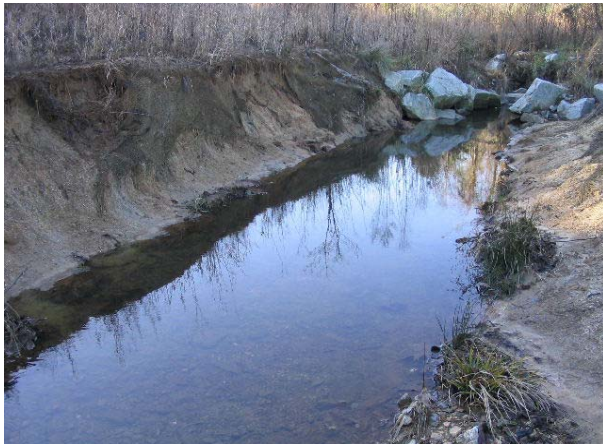
Issue Photo 5 - Station 2+40 Eroding streambank, coir matting ripped, and inadequate vegetation
