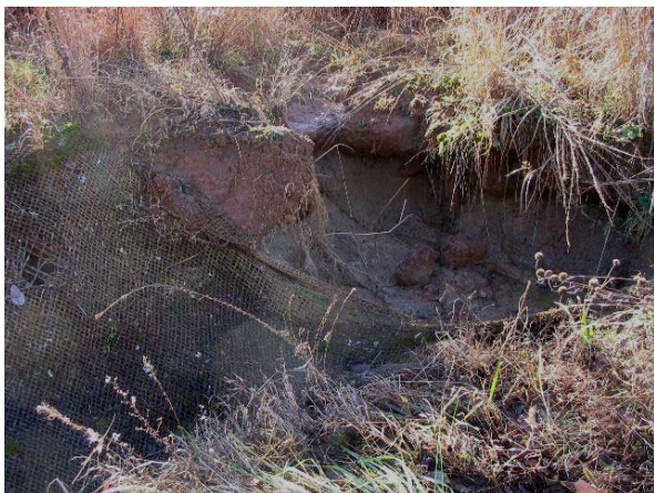
Issue Photo 11 - Station 14+00 Right bank un-vegetated and scoured
