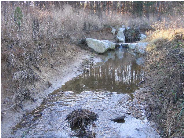
Issue Photo 6 - Station 3+20 Poor vegetation establishment on right bank
