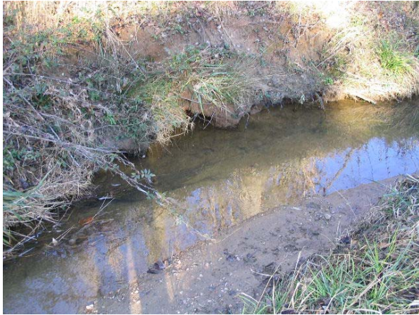
Issue Photo 7 - Station 3+90 Outside meander slump resulting from overland flow
