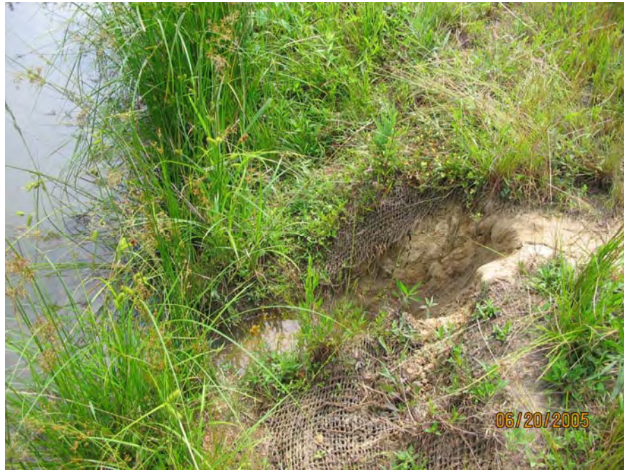
P19. Bank Erosion
