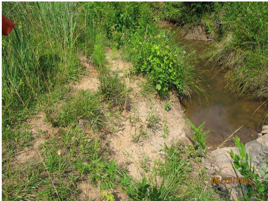
P3. Bank Erosion
