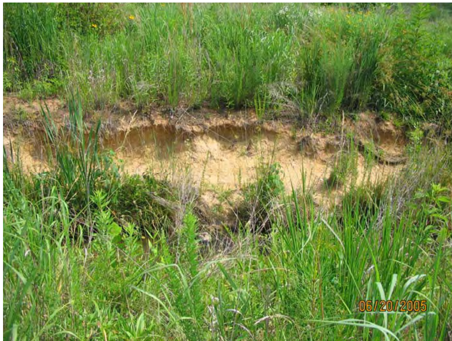
P12a. Bank Erosion
