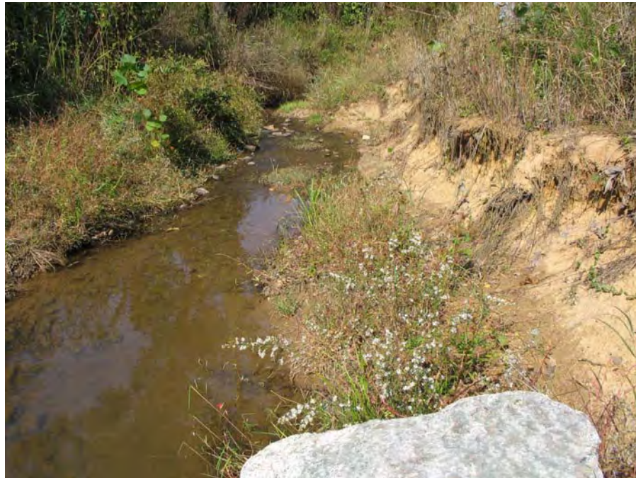
P2. Bank Erosion
