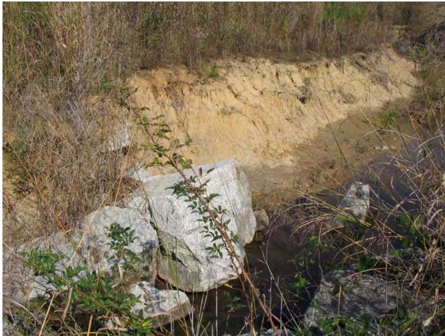
P4. Bank Erosion
