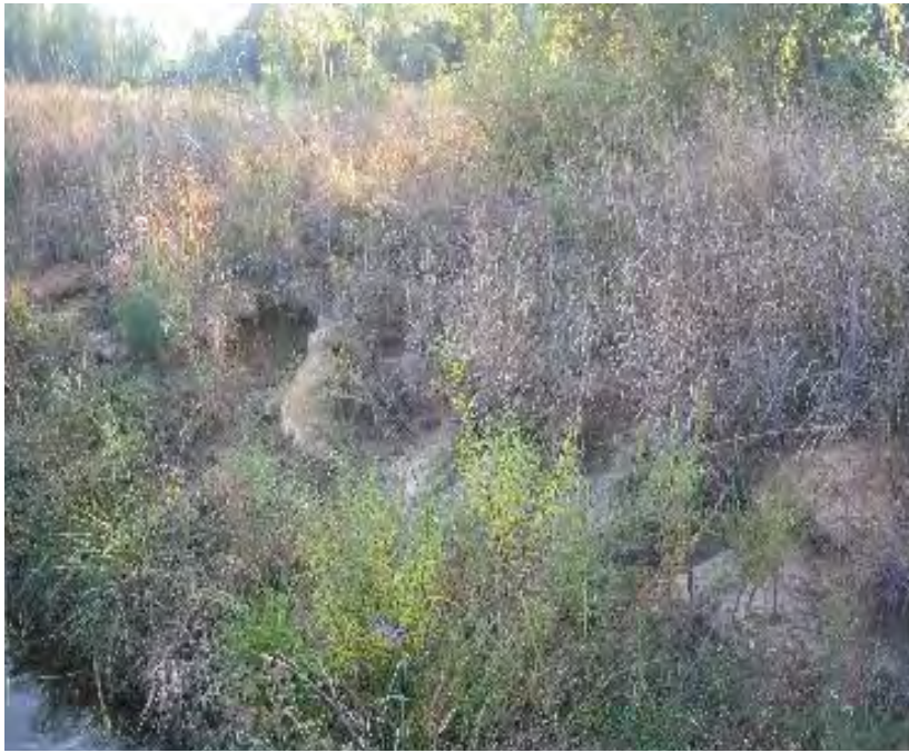
P8. Bank Erosion
