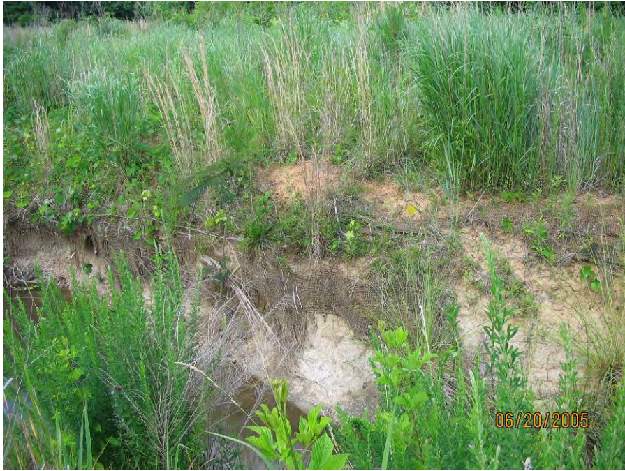
P6. Bank Erosion
