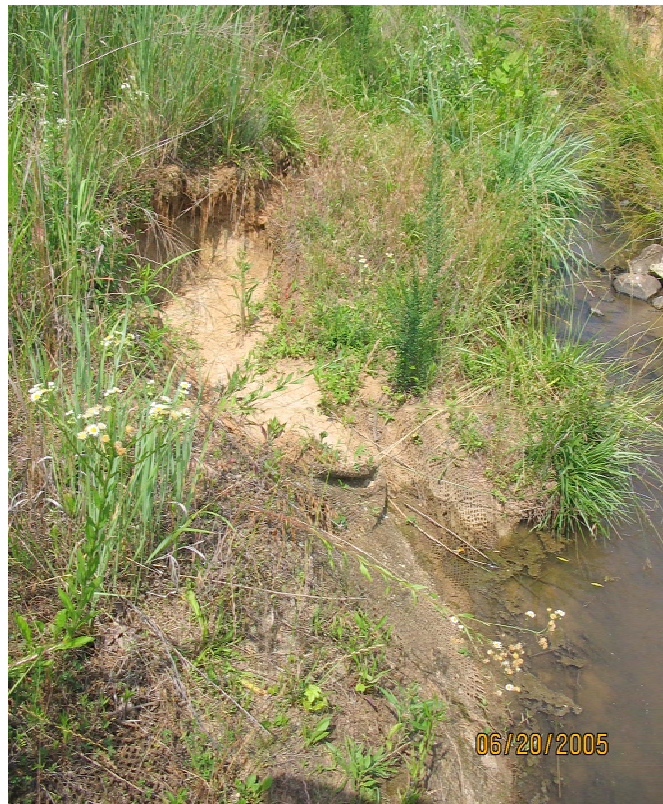
P18b. Bank Erosion
