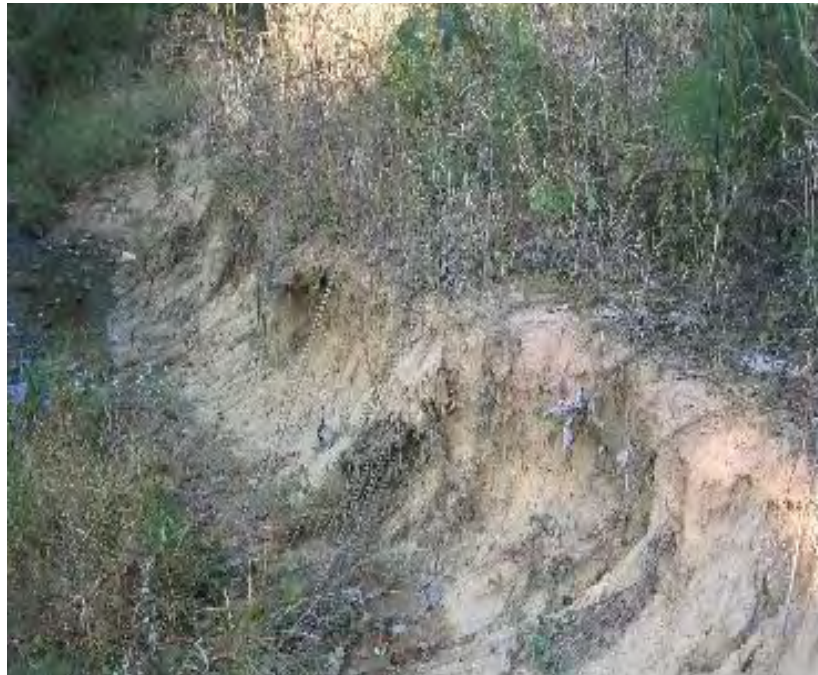
P10. Bank Erosion
