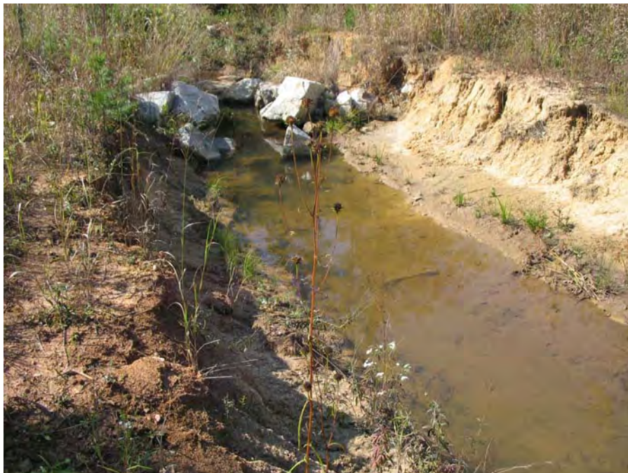
P7. Bank Erosion
