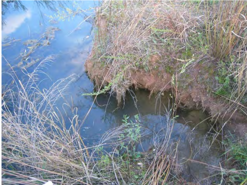
P18a. Bank Erosion
