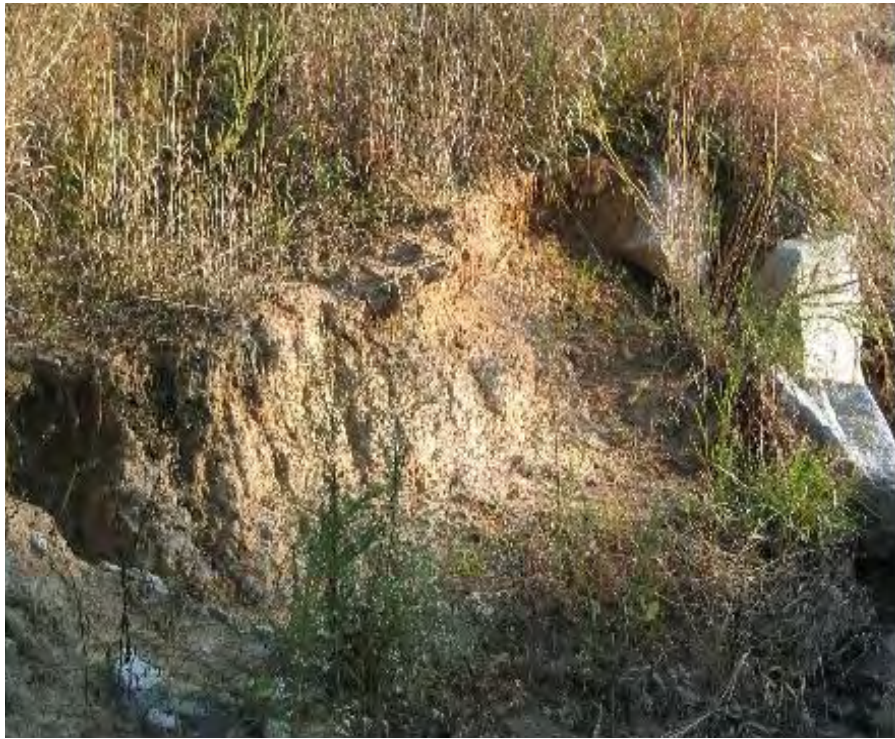
P15. Bank Erosion
