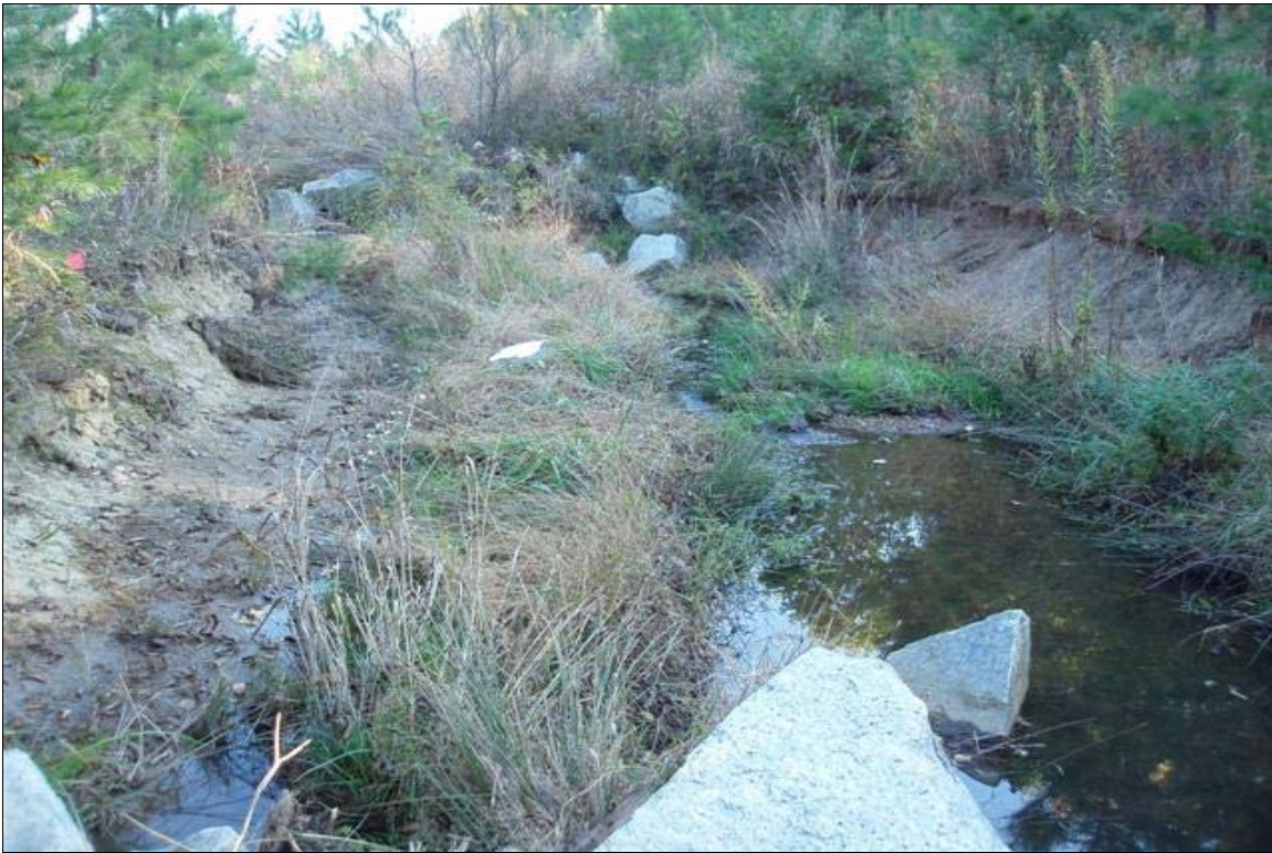
SP1 – Severe bank erosion. Photo taken near Station 4+00 (XS1). 10/29/08 - MY 06
