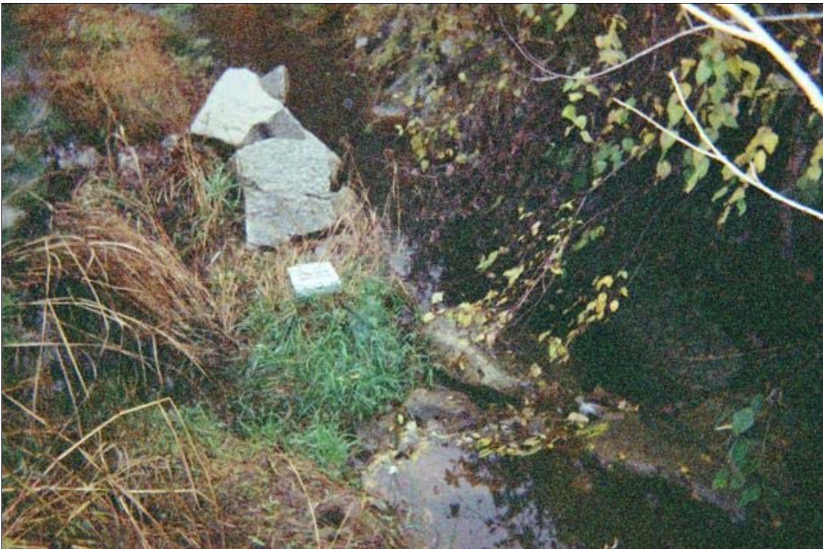
SP4 – Failed cross vane. Photo taken near Station 4+00. 11/5/08 - MY 06
