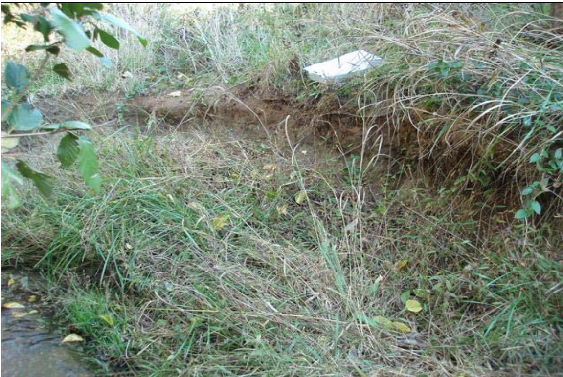
SP2 – Upper bank erosion. Photo taken near Station 5+00. 10/29/08 - MY 06
