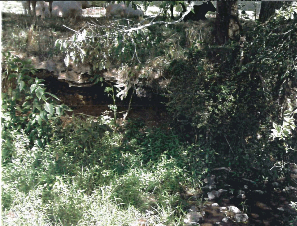
Photo 4: Looking upstream from right bank to left bank at bank undercutting of reach 2
