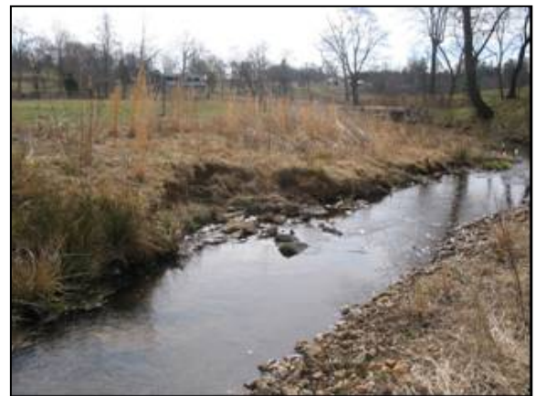
IP 44 Bank Erosion (Station 7+50)
