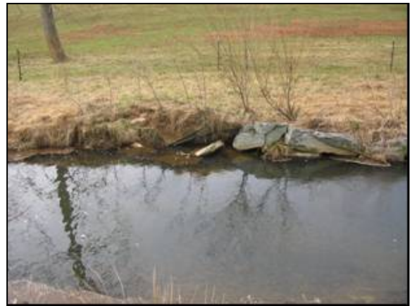
IP 38 Vane Slump and Erosion (Station 1+00)
