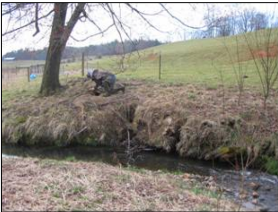
IP 20 Erosion Ground Hog Tunnels (Station 4+00)
