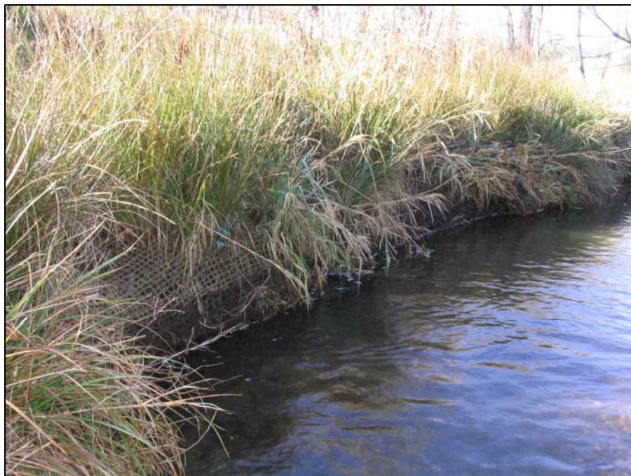
IP1. Reach 1 – Station 5+75 Eroding Bank (Oct. 5, 2007) (top photo looking upstream, bottom photo looking downstream)
