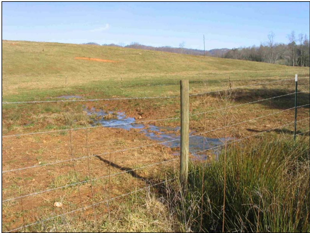
IP2. Reach 1 – Station 9+80 – Concentrated flow into and through the buffer. (Oct. 5, 2007) (top photo – gully through buffer. Bottom photo – seep from field)
