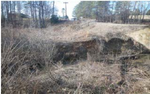
Photo 1. Area of bare bank at utility crossing at top of project on mainstem.
