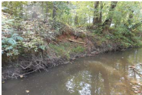
Photo 2. Area at Station 16+00 called a Vegetation Problem Area in past but has been stable over the last two years even though a small area of bare bank remains.
