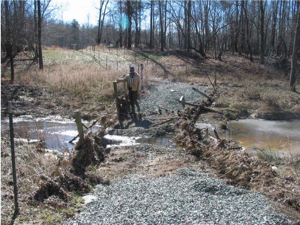
Photo 4. Storm damage to cattle crossing fence.
