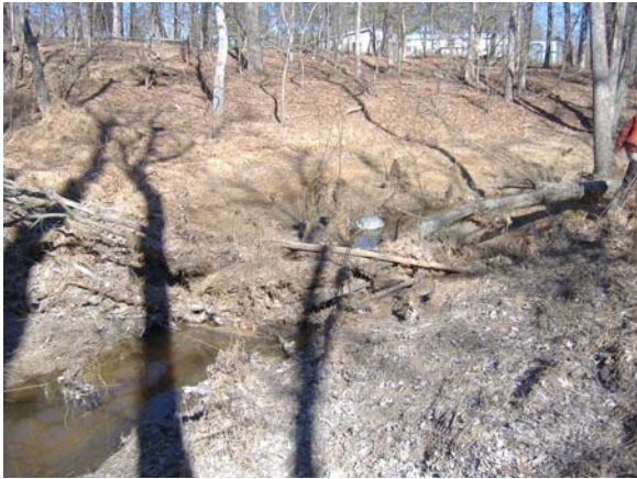
Photo 7: Representative debris jam (Station 34+73 along plan view).
