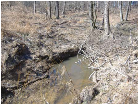
Photo 3: Representative bank erosion problem area (Station 35+98 along plan view).
