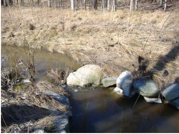
Photo 5: Representative problem crossvane (Station 29+88 along plan view).
