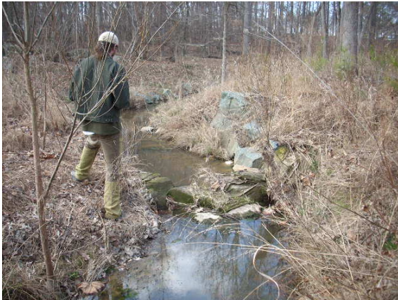
Photo 3: Representative cross-vane problem area (Station No. 32+85; view downstream; 2-25-2008).
