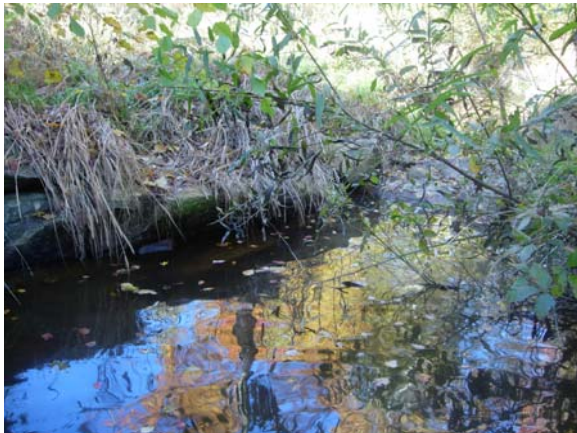
Photo 7: Representative problem jhook; Piping is occurring around right arm of j-hook (Station No. 13+07, view upstream on 11-6-2008).
