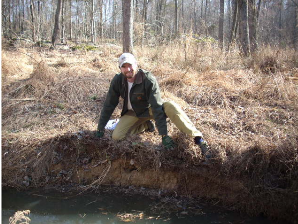
Photo 1: Representative bank erosion problem area (Station No. 24+29; view of right bank; 2-25-2008).
