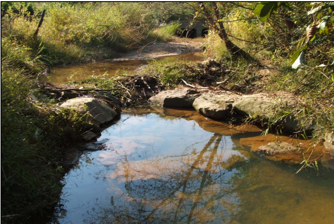
Photo Station 8 (Reach 2) – View looking upstream at rock cross vane, note loss of back fill material in front of cross vane arm on right side of photo.
