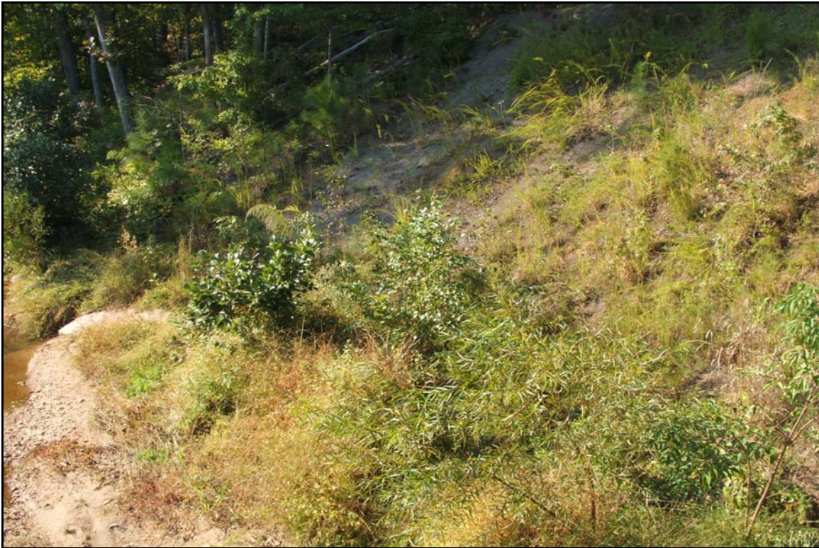
Photo Station 1 (Reach 1) – View looking southwest at the left bank and the slope above.
