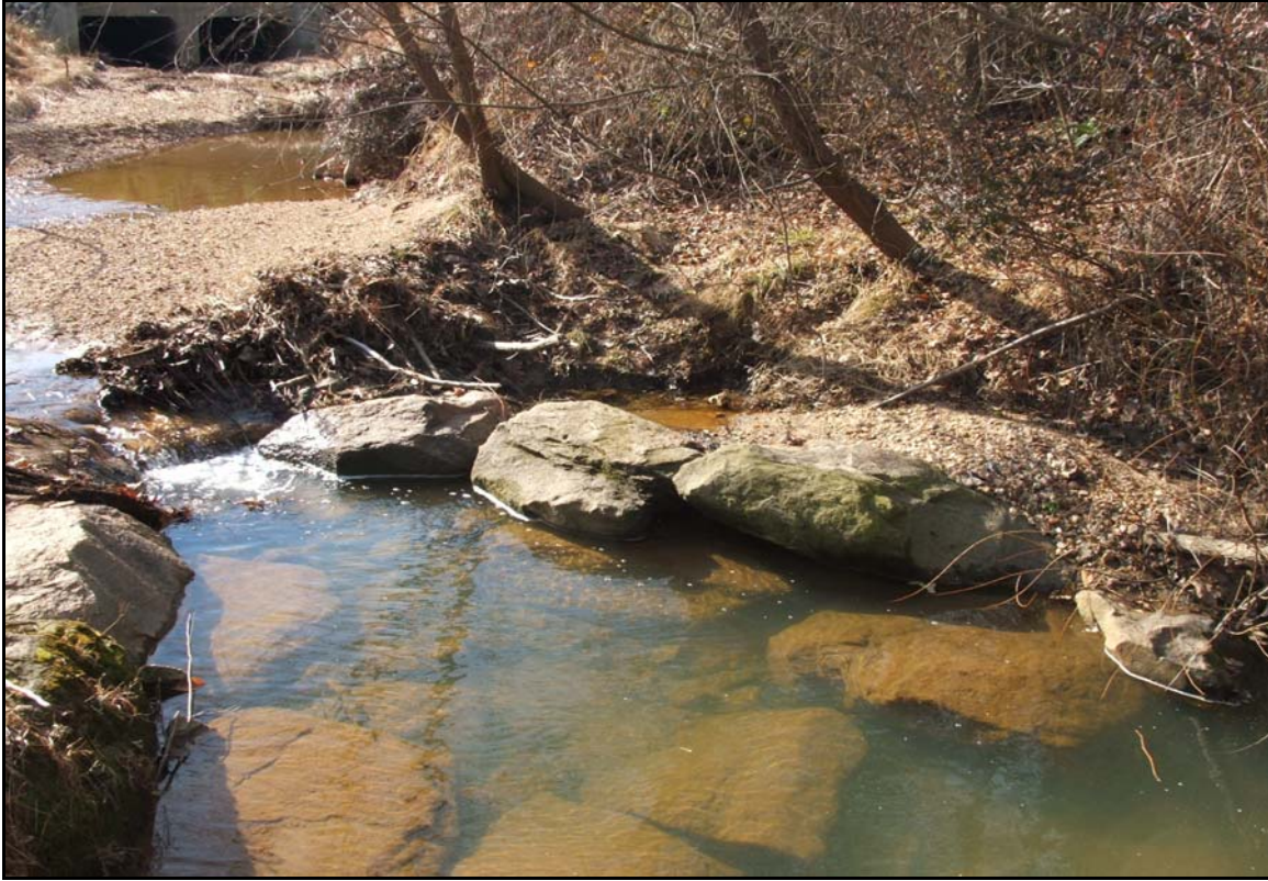
SP 1 (Reach 2) – Back arm scour on left arm of cross vane.
