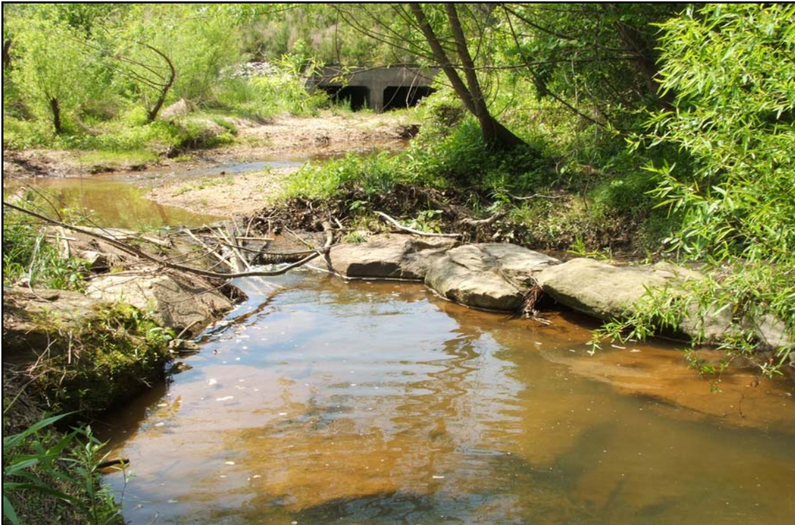
Photo Station 8 (Reach 2) – View looking upstream at rock cross vane, note loss of back fill material in front of cross vane arm on right side of photo.
