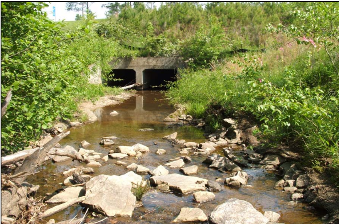
Photo Station 2 (Reach 1) – View looking downstream with culvert under Collector Rd. in center of photo.
