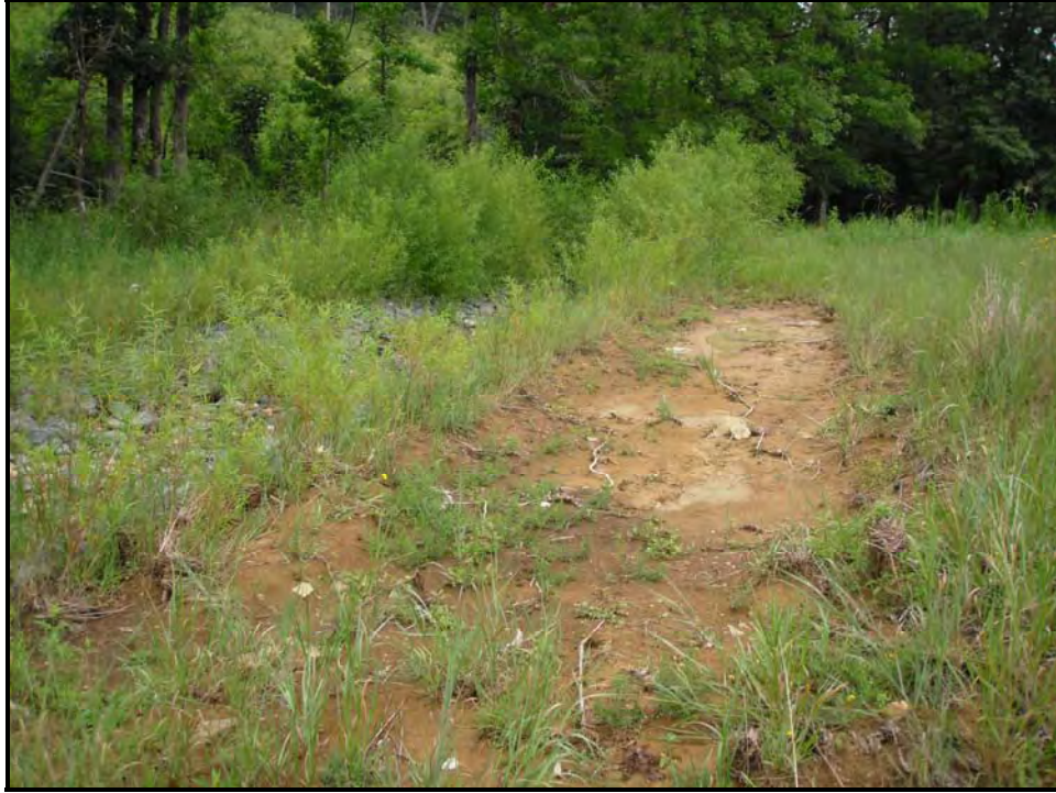
SPA # 3. Right bank erosion at Sta. 168+50.
