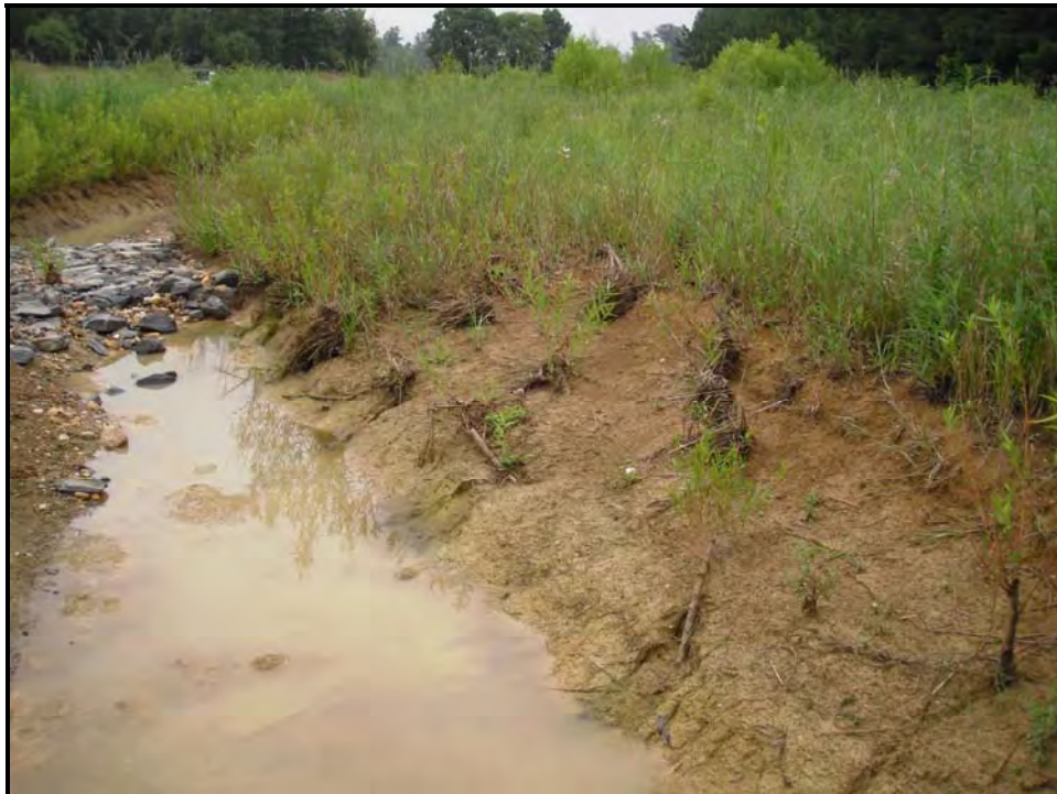
SPA # 2. Minor right bank erosion at Sta. 149+50.
