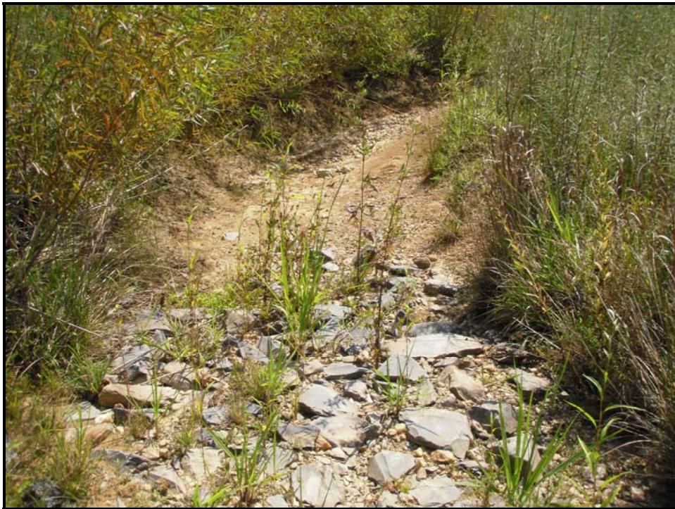
SPA # 2. Minor right bank erosion at Sta. 149+50.
