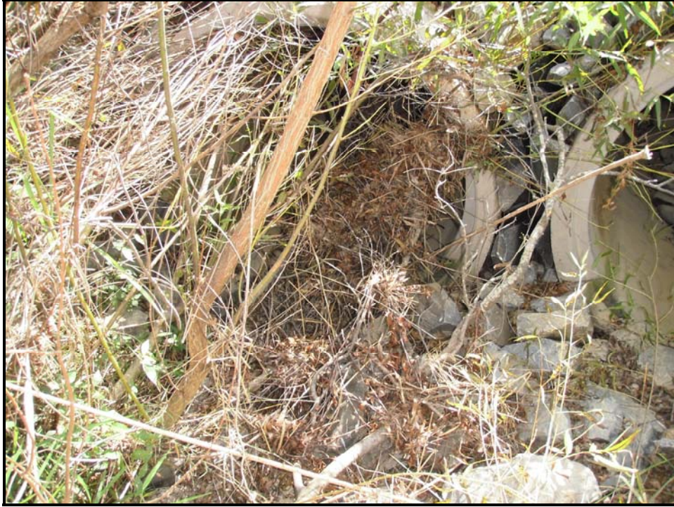
SPA # 1. Culvert blocked by debris at Sta. 140+25.
