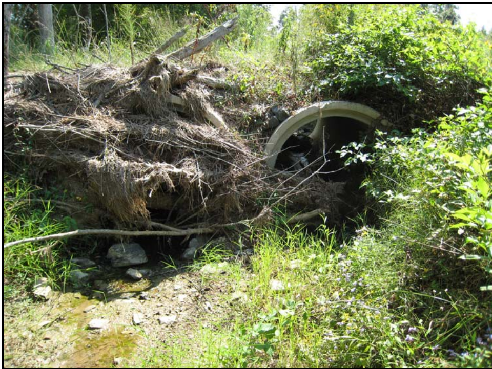
SPA # 4. Culvert blocked by debris at Sta. 172+00.
