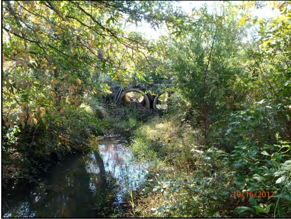
SPA # 3. Culvert blocked by debris at Sta. 172+00.
