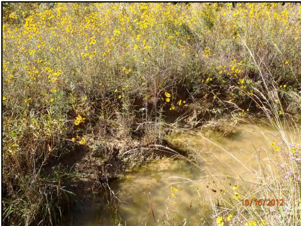
SPA # 2. Minor right bank erosion at Sta. 149+50.
