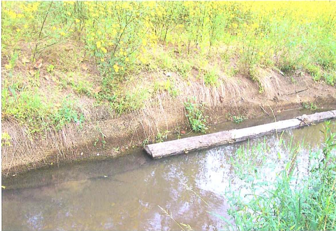
Rocky Branch, (Stations 23+70 – 23+90) Stretch of channel with sloughed banks. View looking across channel from right to left.
