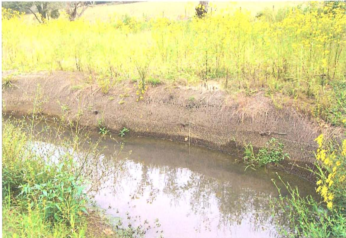
Rocky Branch (Stations 34+00 – 34+30) Area of sloughing banks. View looking across channel from left to right.
