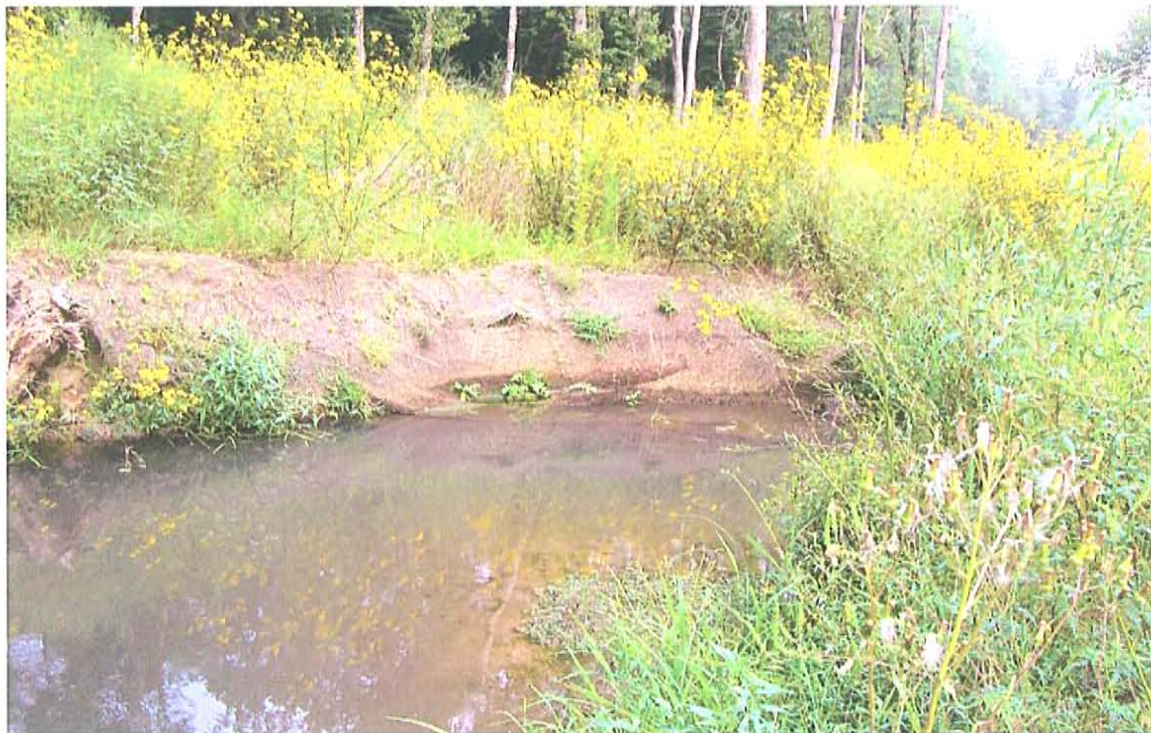
Rocky Branch, (Stations 25+70 – 25+80) Stretch of channel with sloughed banks. View looking across channel from right to left.
