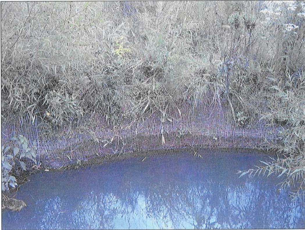
STREAM PROBLEM AREA 5: ROCKY BRANCH (STATIONS 34+00 - 34+30) AREA OF SLOUGHING BANKS. VIEW LOOKING ACROSS CHANNEL FROM LEFT TO RIGHT.
