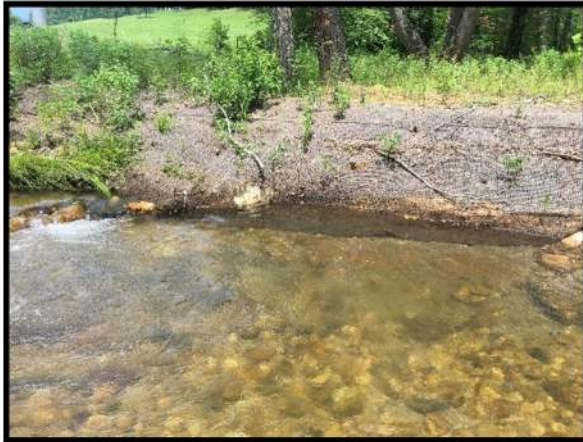
3.21 Minor erosion at rock step structure STA 37+27 (Roses Creek)
