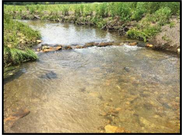
3.20 Scour below rock step structure STA 37+25 (Roses Creek)
