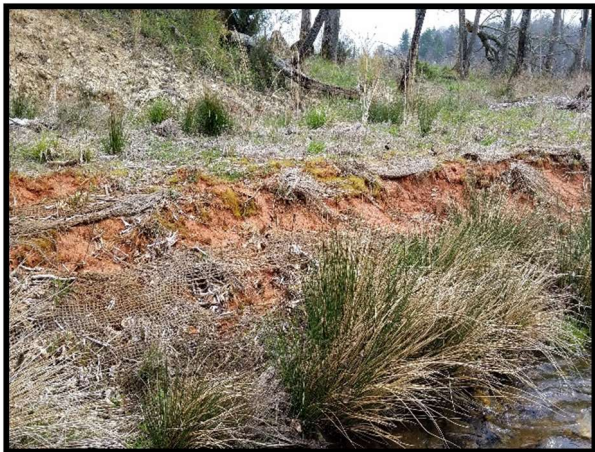
3.20 Erosion at station 12+69-12+91
