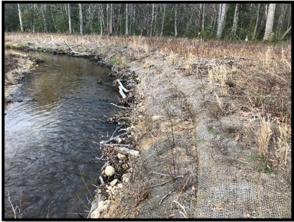
3.26 Erosion at station 39+26-39+44
