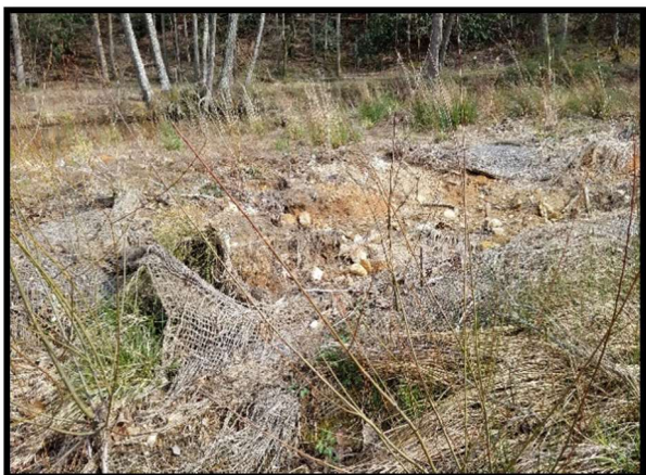
3.22 Erosion at station 35+90-36+18
