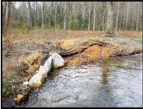
3.24 Severe Erosion and rock step at station 37+10-37+30
