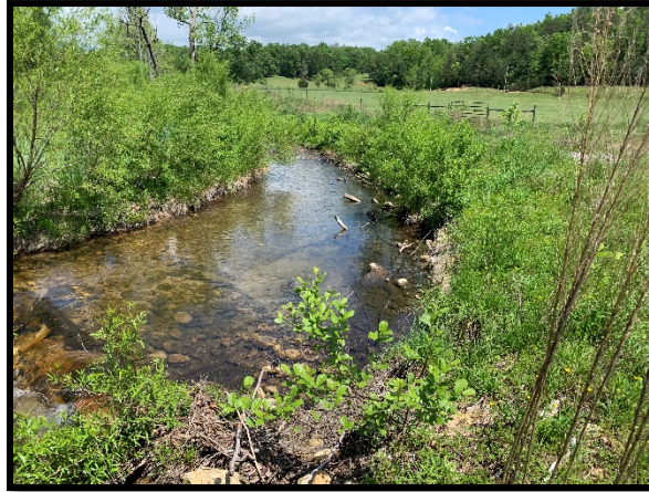
3.2 Minor erosion at 20+10
