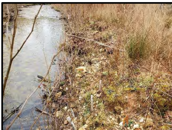
3.23 Minor erosion at station 35+00.
