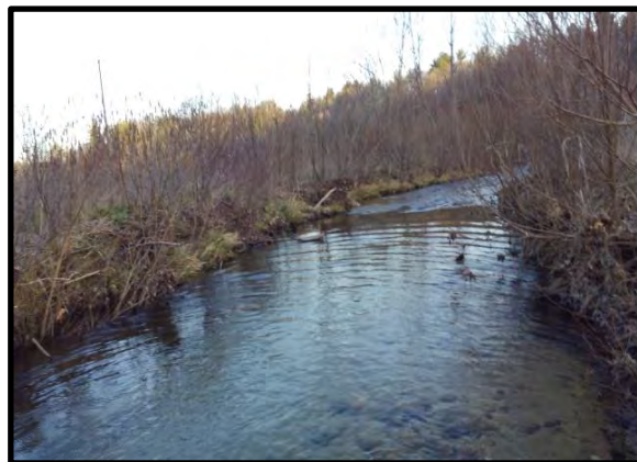
3.18 Minor erosion at station 20+00
