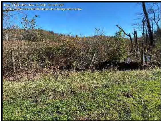
3.27 Damage to fence from October rain events.
