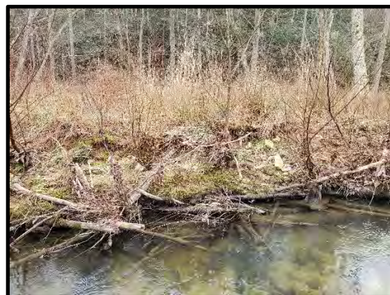
3.24 Minor erosion at station 39+30.
