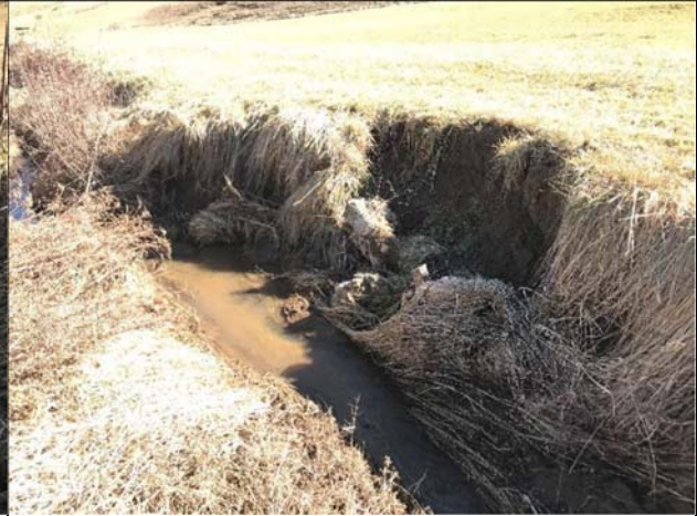
Photo 8: Looking at RHB-2 unstable and slumping banks.
