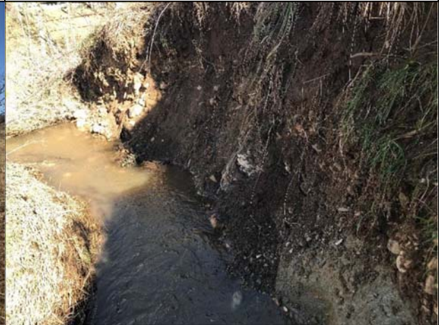
Photo 10: Looking at bank erosion along the right bank of RHB-3 near the end of the property.
