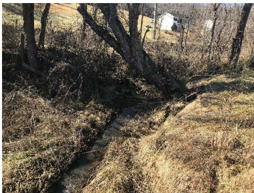
Looking upstream at the old roadbed and culvert in T1 causing a blockage.
