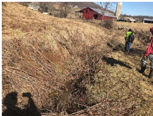
Bank erosion at outer left bend as RHB-1 attempts to adjust laterally upstream of the ford crossing.
