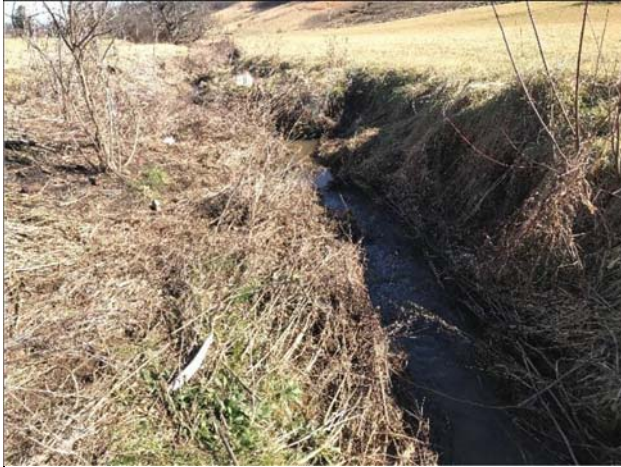
Photo 7: Looking at RHB-2 downstream of the confluence with T1 and the driveway culvert.
