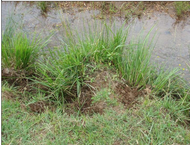
View looking east at Tributary 1 from the top of the project reach. Erosion is channelizing and incising the stream. 6/4/15
