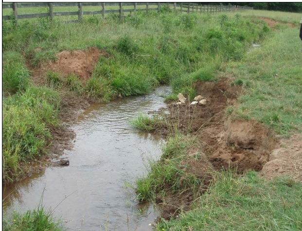
View looking southeast and downstream at bank erosion midway through the length of T1. 6/4/15
