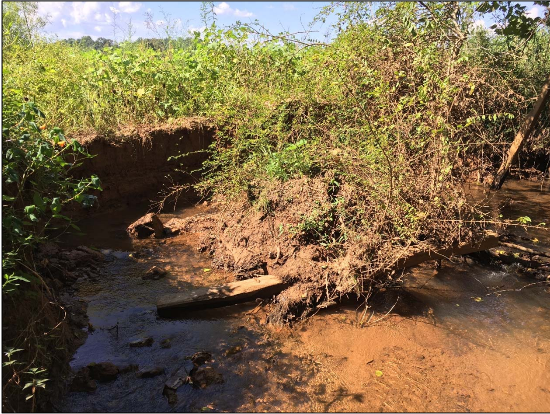
Photo 1. Eroding stream bank that was encroaching into easement before repair, 8/29/2018
