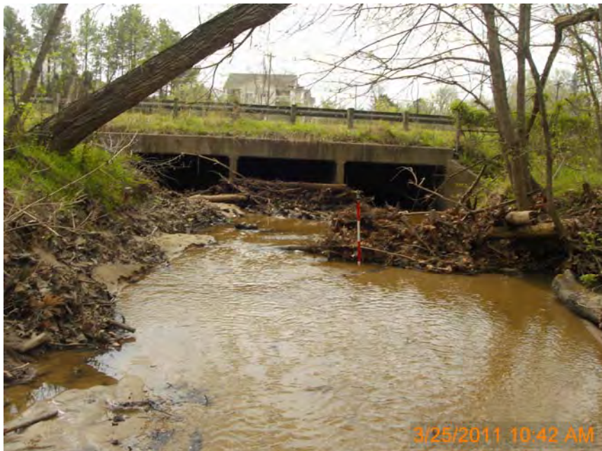
Culverts and Debris (Station 0 + 00)
