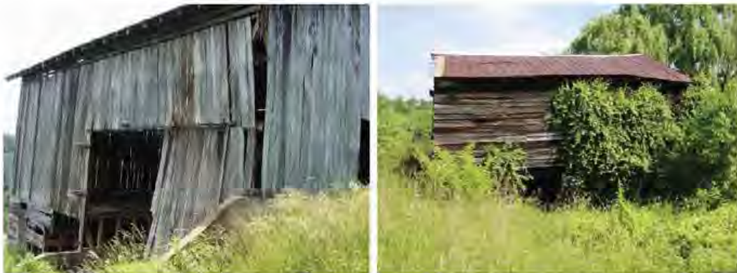
Two of the structures slated for removal from the game land are the Don Snellson- second barn (left) and the Martin Candler barn (right). Pictures above are from several years ago and since then both structures have become even more dilapidated and pose a potential liability to the public.
