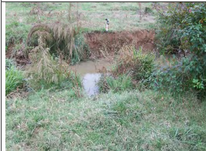
Photo 5- View of UT1 left bank erosion at XS 10.
