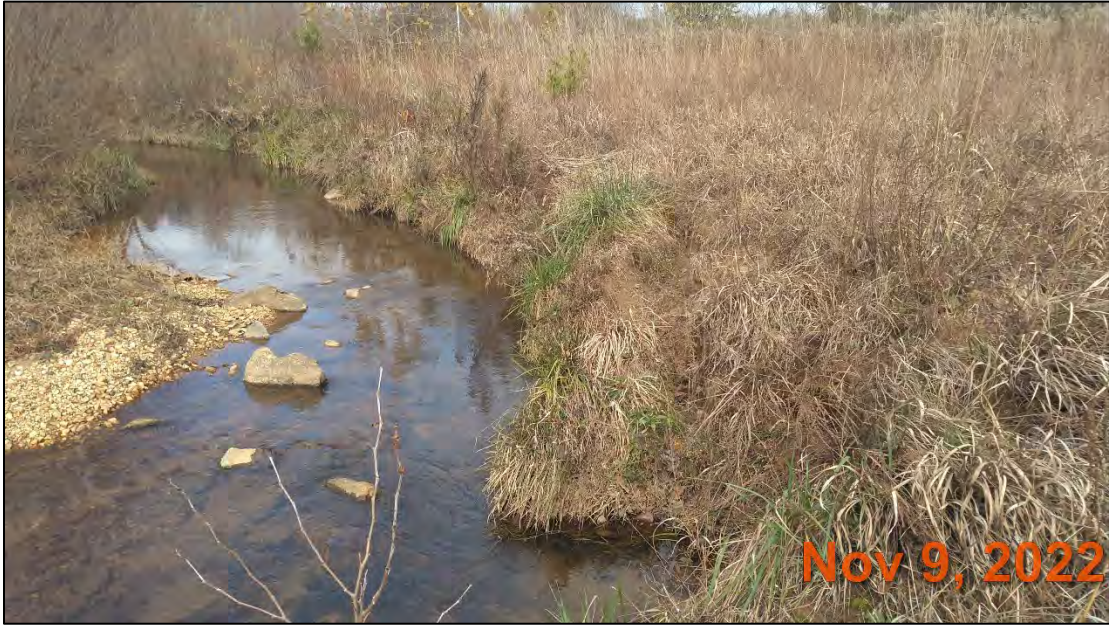
Bank Slump, Shadrick Reach 3, Station 113+75
