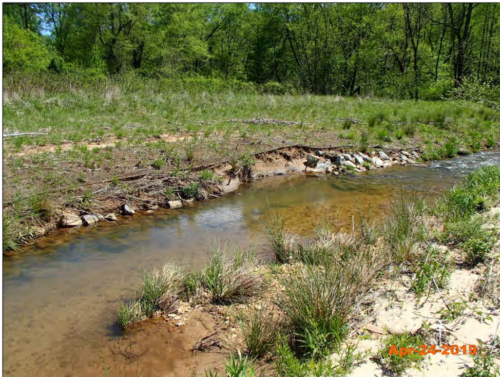
UT1– Bank Erosion Station 29+50
