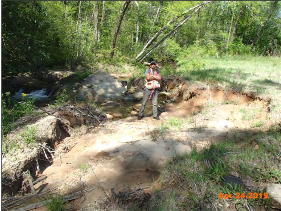
Shadrick Creek Reach 1 – Bank Erosion Station 11+00
