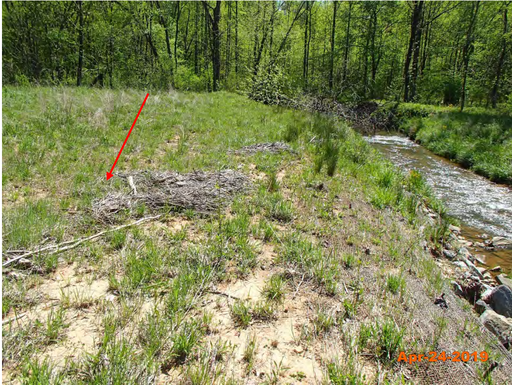
Photo #3 – Shadrick Creek Reach 3 STA 115+50 Wrack Lines
