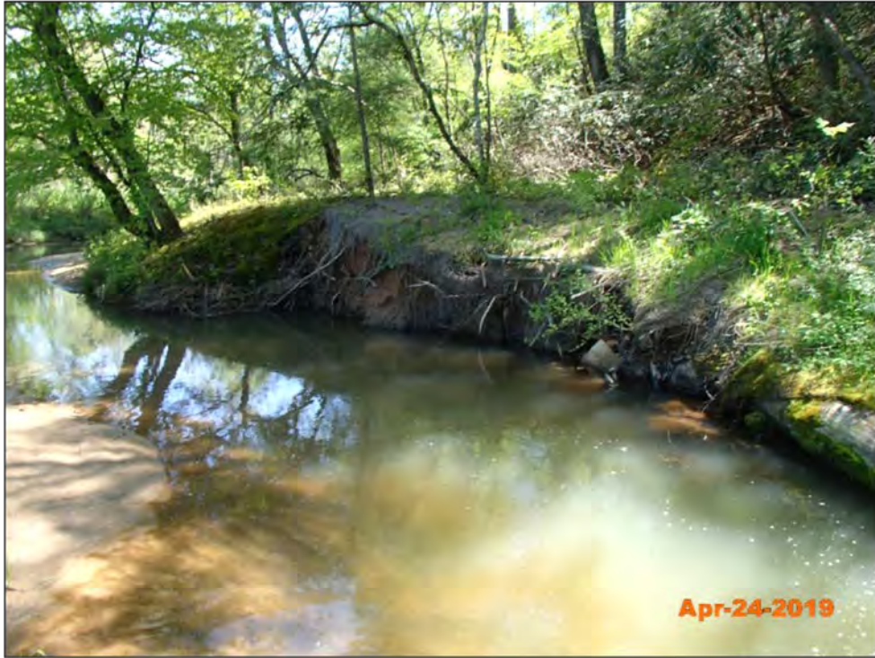
Shadrick Creek Reach 1 – Bank Erosion Station 37+50
