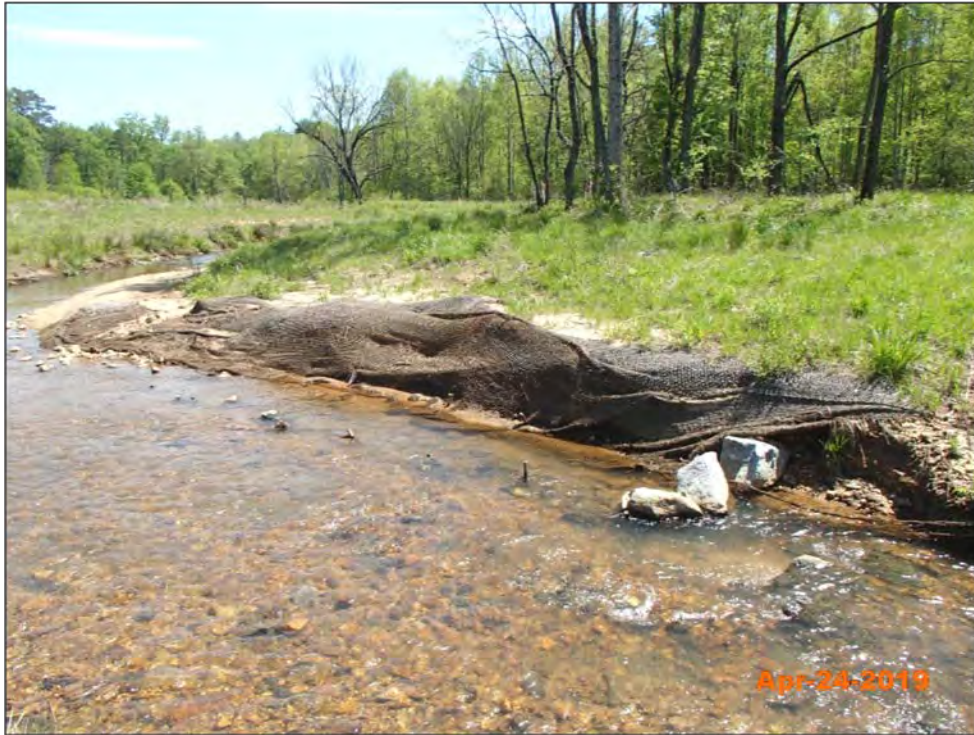
Shadrick Creek Reach 3 – Bank Erosion Station 107+50
