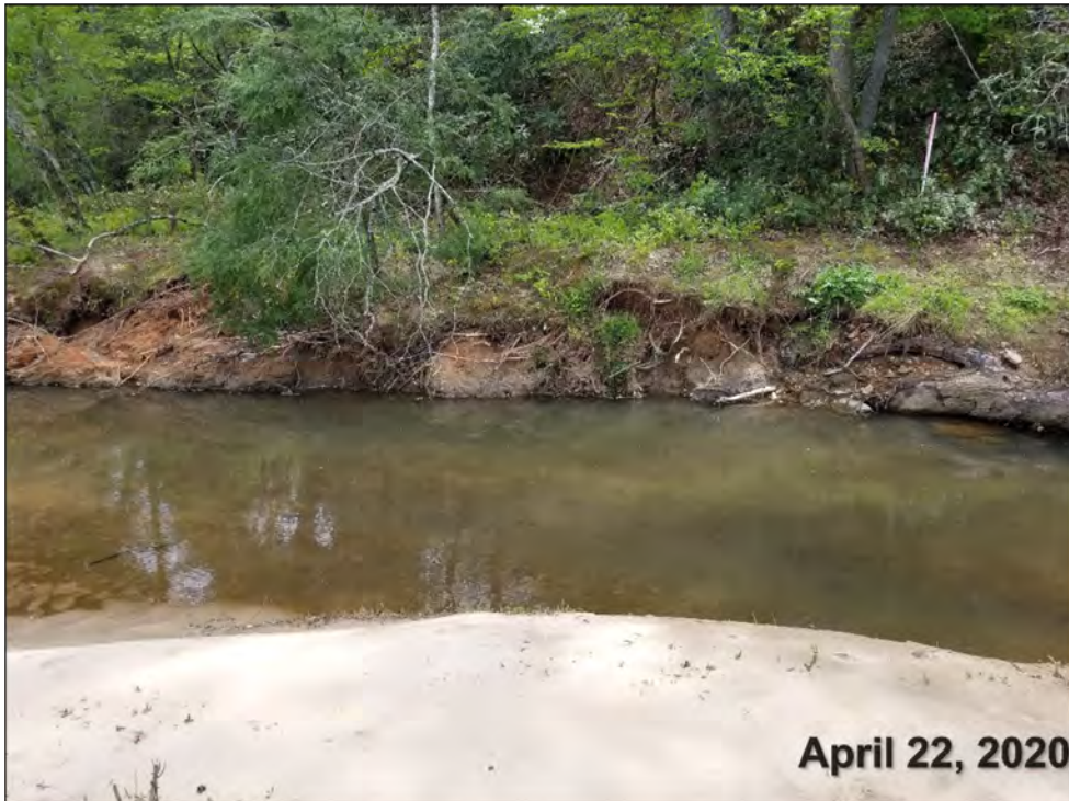
Shadrick Creek Reach 1 – Bank Erosion Station 37+50
