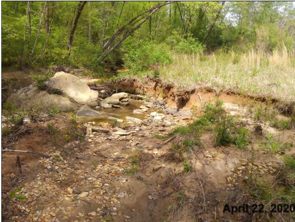
Shadrick Creek Reach 1 – Bank Erosion Station 11+00
