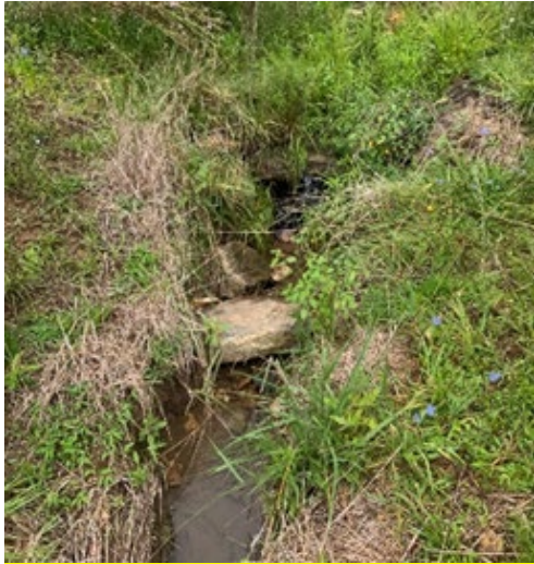
UT3 Reach 2 STA 306+00: typical headcut, structure piping
