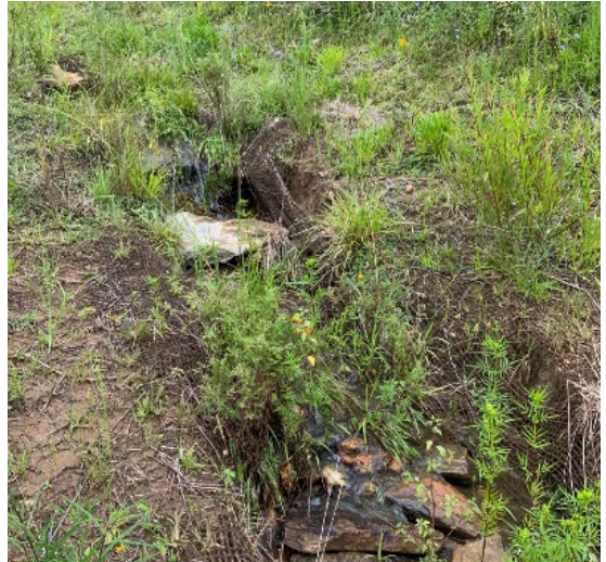
UT3 Reach 2 STA 307+75: typical bank instability
