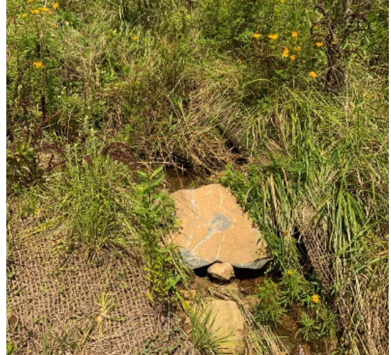
UT4 STA 404+25: Typical headcut, structure piping
