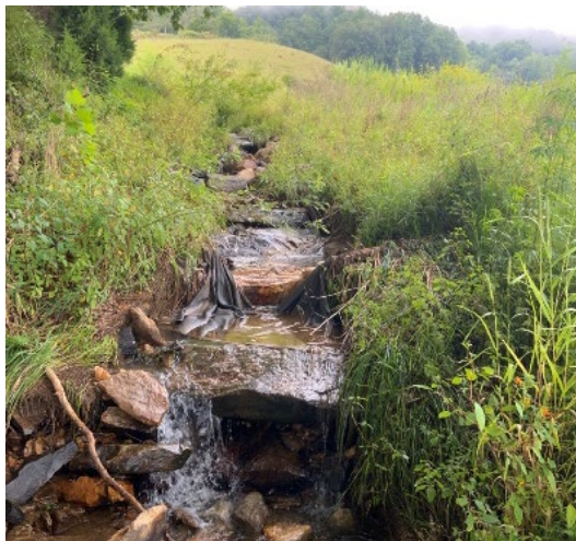
Shake Rag Reach 3 STA 921+50 & 921+75: Typical bed and bank instability
