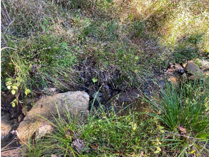
UT1 Reach 2 STA 112+00: headcut due to structure piping
