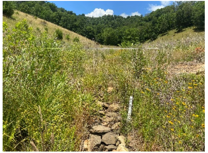
UT3 Reach 2 STA 312+00: typical bed instability
