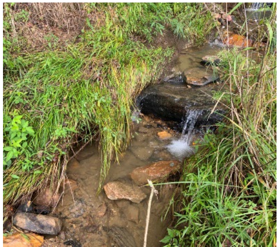
Shake Rag Reach 3 STA 922+15: Typical minor bank instability
