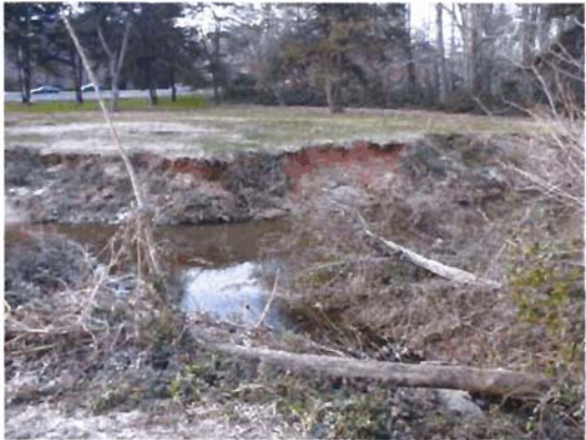
I. Bank Erosion on Silas Creek
