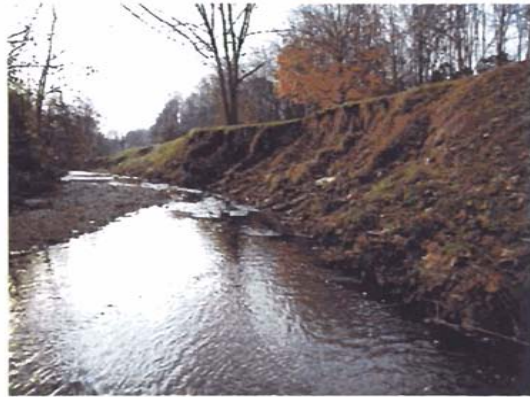
K. Bank Erosion on Silas Creek
