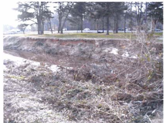
L. Bank Erosion on Silas Creek
