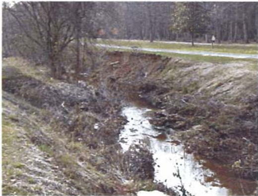
J. Bank Erosion on Silas Creek
