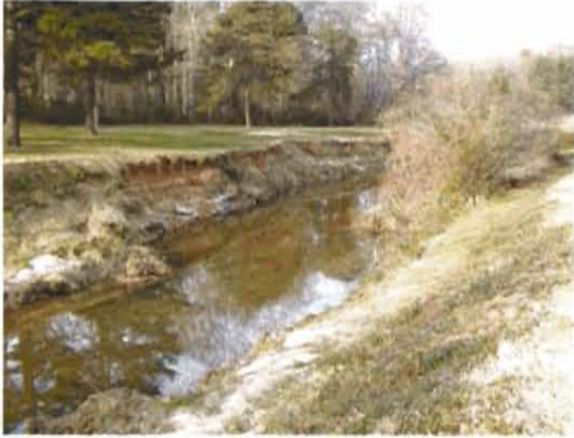
M. Bank Erosion on Silas Creek
