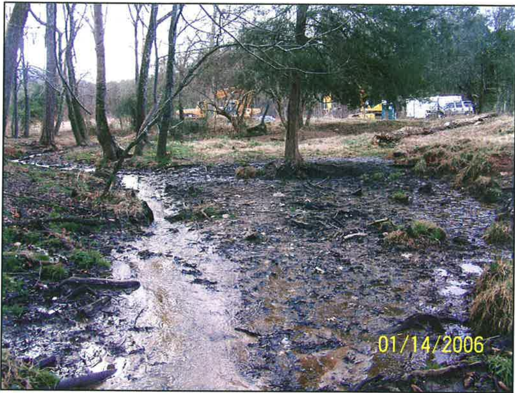
5. Evidence of extreme cattle intrusion and bank failure attributed to hoof shear along Unnamed Tributary at bottom of reach.
