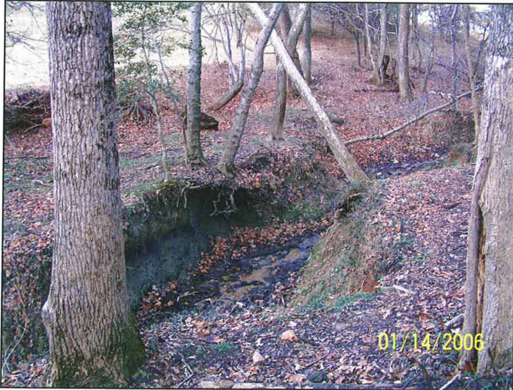
8. Undercutting of banks along Unnamed Tributary is resulting in loss of trees in some areas.
