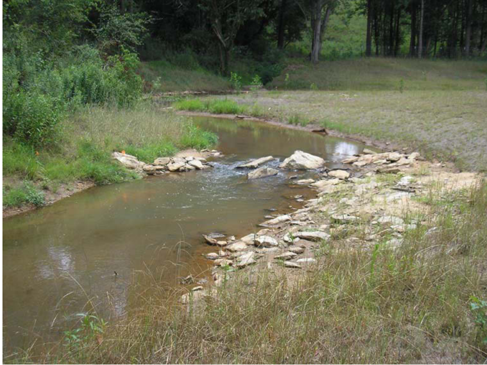
J-Hook Rock Vane – Looking Upstream at the confluence of UT-D – Post Restoration
