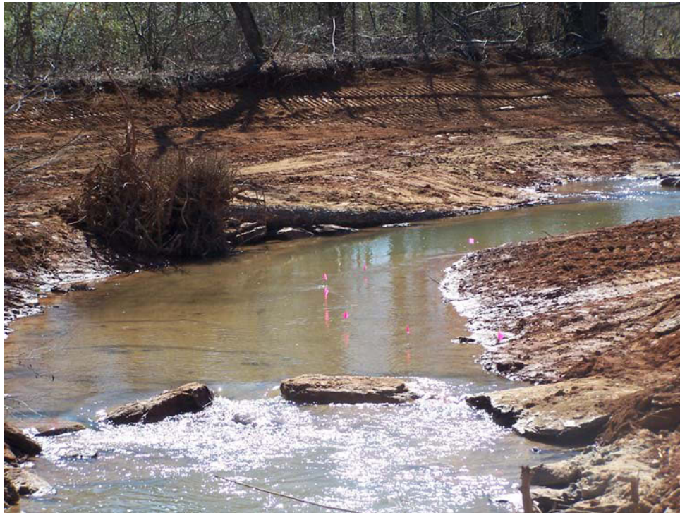
Bottom of Mainstem Reach – Log-Vane, J-Hook, Root Wad Combination Structure followed by Cross-Vane No. 4 – During Construction - End of Mainstem Project
