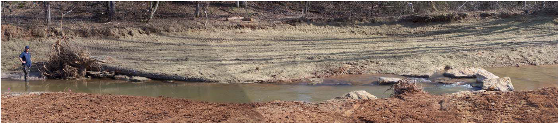
Mainstem Reach – Log-Vane, J-Hook, Root Wad Combination Structure – After Seeding, Mulching and Jute Matting Right Bank – February 2007
