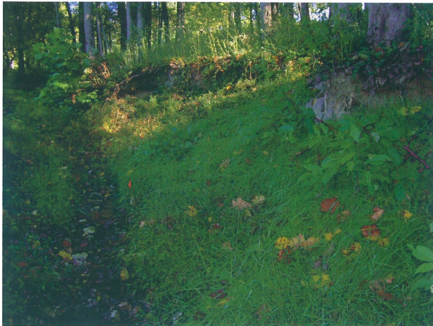
SPA 2 Steep banks in need of stabilization along Unnamed Tributary A near station 13+00. (EMH&T, Inc. 10/22/07)
