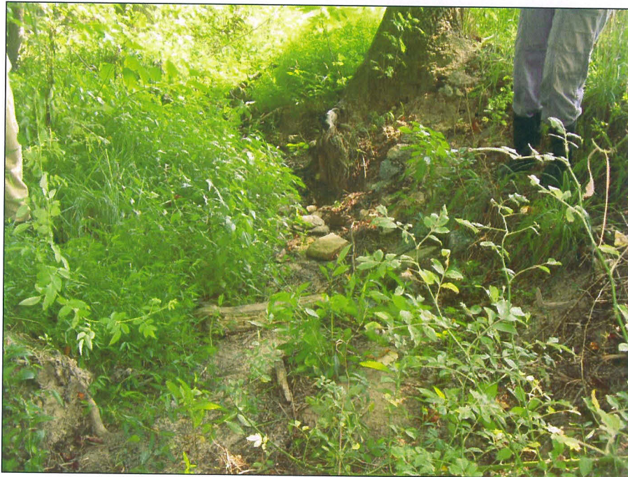
SPA 2 Right streambank scour on Unnamed Tributary A near station 3+55. (EMH&T, September 8, 2008)
