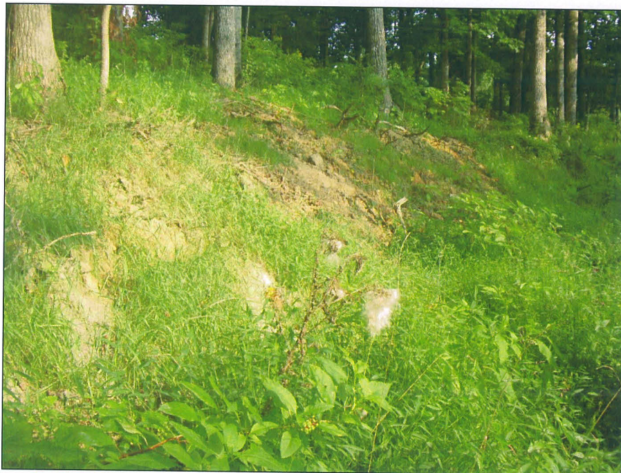
SPA 4 Steep streambanks on Unnamed Tributary A, looking downstream near station 12+00. The streambanks have been mechanically reshaped; the remaining stabilization will occur using vegetative means. (EMH&T, September 8, 2008)
