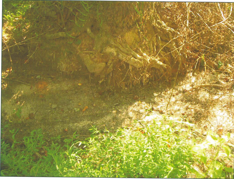
SPA 3 Close-up of right streambank scour on Unnamed Tributary A near station 3+55. (EMH&T, September 8, 2008)
