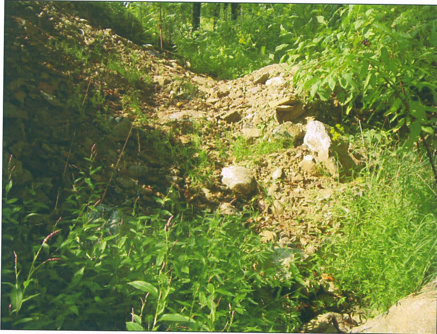
SPA 1 Natural log sill on Unnamed Tributary A near station 5+75. Log sill was removed and channel stabilized with rock. (EMH&T, September 8, 2008)
